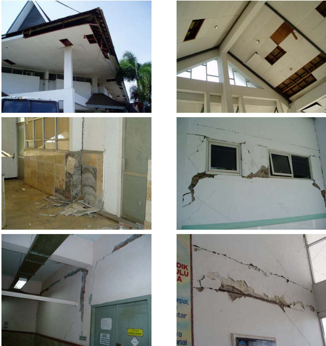
Figure 4.: Non-structural damage at M. Yunus hospital, Bengkulu
