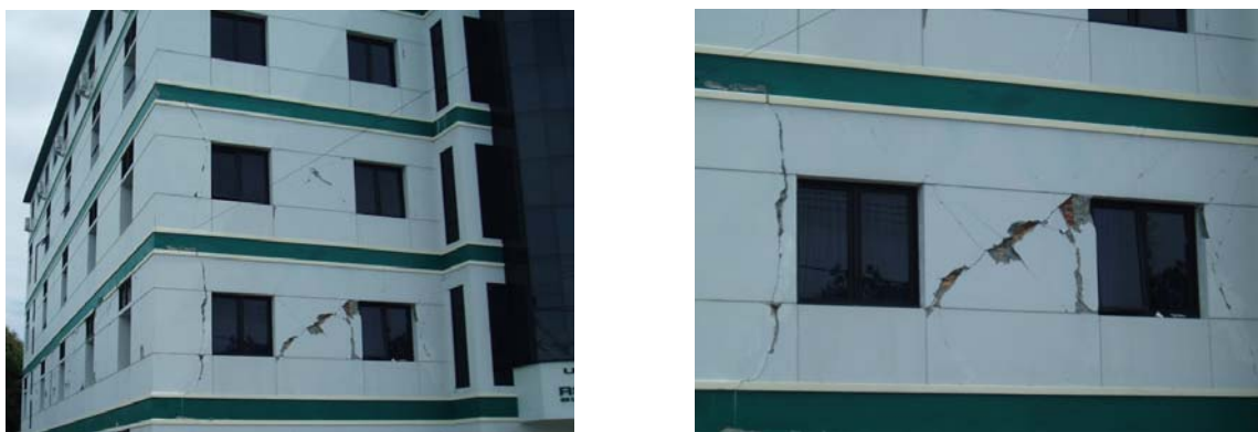
Figure 5.: Non-structural damage at Bunda Medical Center hospital, Padang, West-Sumatra
