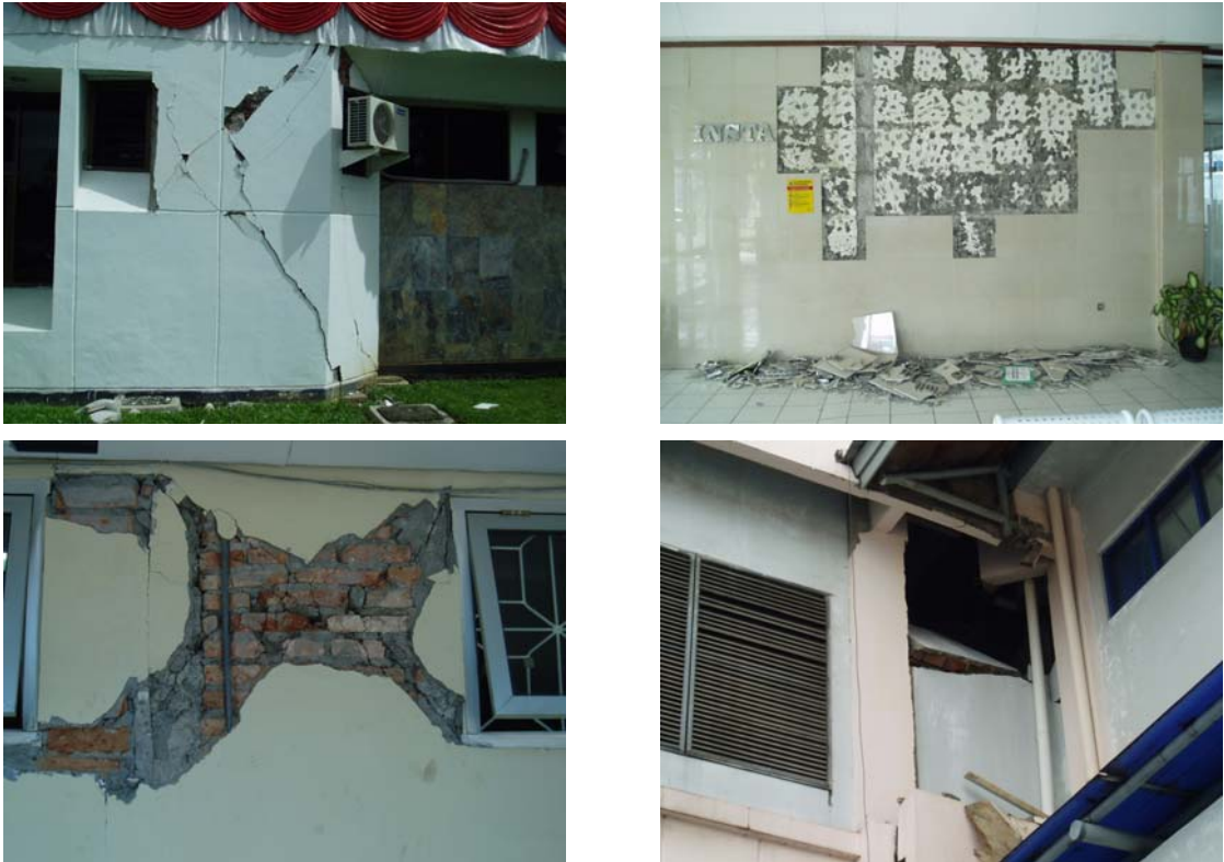
Figure 6.: Non-structural damage at M. Djamil hospital, Padang, West-Sumatra
