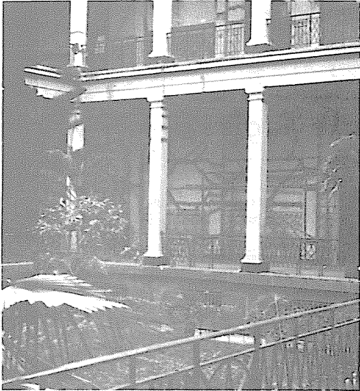
All walls of the three floors facing the courtyard were cracked, as were the perimeter columns.
