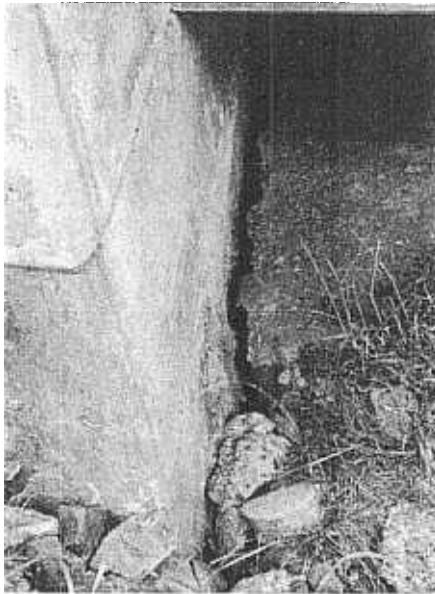
Soil movement at the Lindley Bridge abutment
