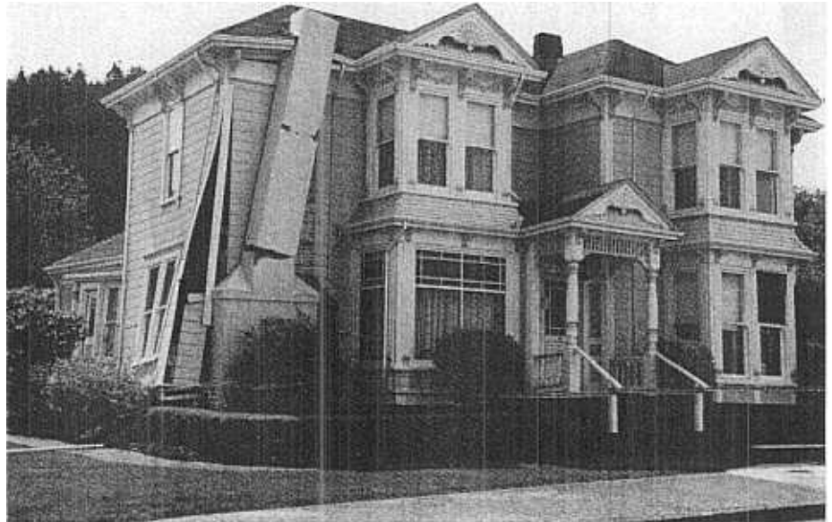
Damage to a Victorian house in Ferndale
