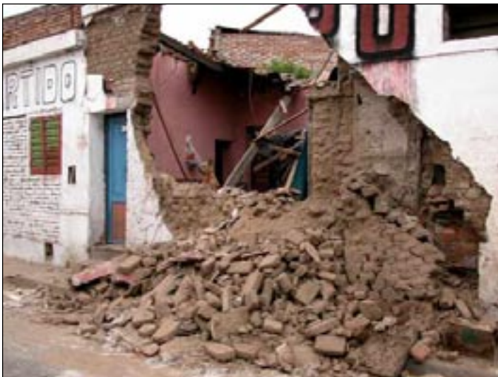
Damage to adobe structure in Catamarca (photo: El Diario Clarin).
