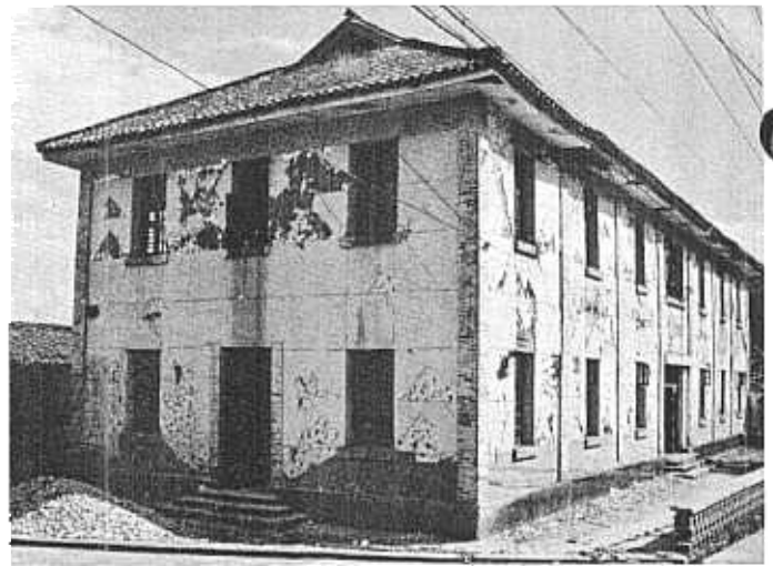
Photo 2. Administrative building of Gengma County. Adobe walls with brick piers. Intensity 8.
