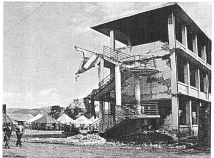
Photo 6. Yansoi Village middle school, after earthquake shaking intensity 9. Three-storied reinforced concrete frame structure.
