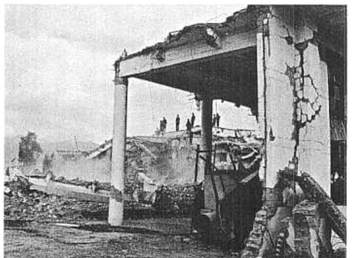
Photo 8. Mingseng tea factory, after earthquake intensity 8. Two-storied reinforced concrete frame structure; top story collapsed.
