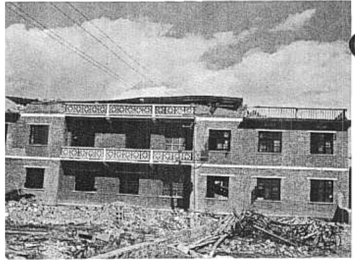
Photo 4. Office building, Gengma County, intensity 8. Three-storied brick masonry structure with monolithic reinforced concrete floors.
