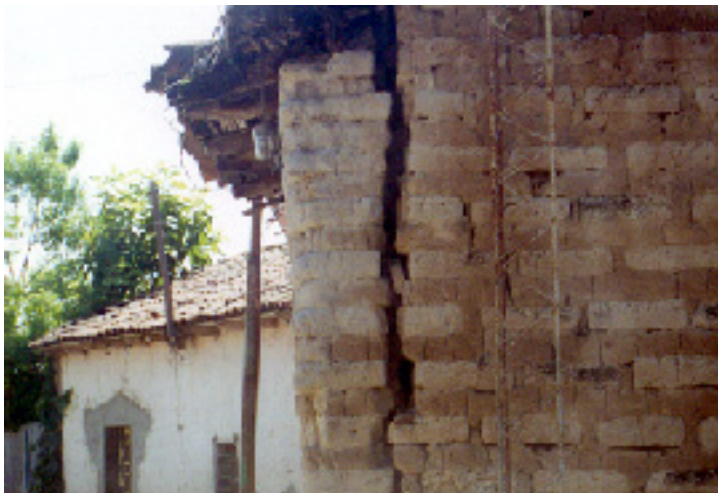
FIGURE 6D: Wall damage (corner separation) in the 1999 Apastepeque earthquake
