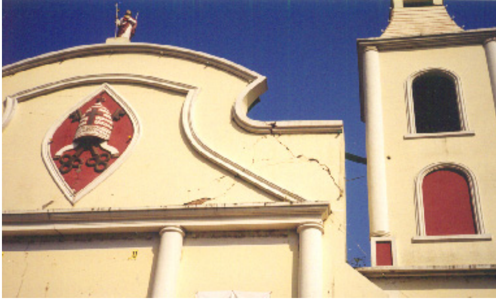
FIGURE 6C: Damage to an adobe church in the 1999 Apastepeque earthquake
