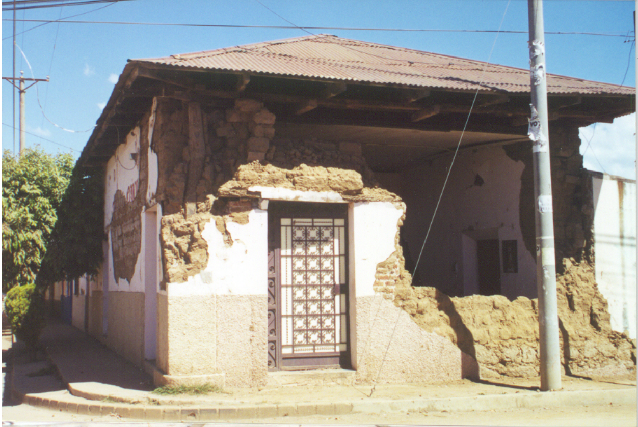
FIGURE 6E: Damages in the town of Juayua due to the January 13, 2001 earthquake
