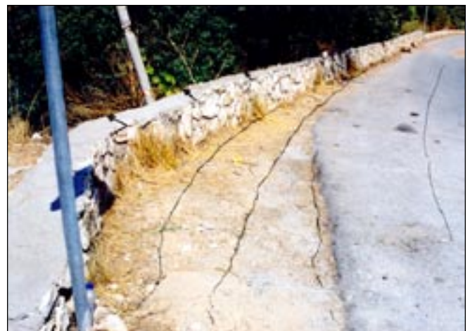
Figure 9. Many retaining walls leaned towards the external side; the adjacent parts of the roads subsided, and cracks appeared on the pavement (NTUA-UoA team).
