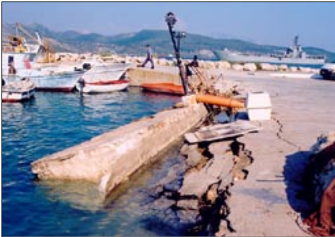
Figure 10. Ground subsidence of the fill material of about 30 cm (NTUA-UoA team).
