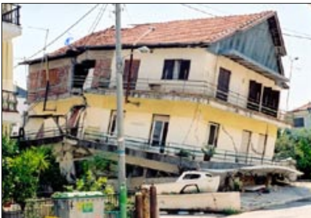
Figure 19. Collapse of R/C building in the town of Lefkada. On the right side, there are no brickwalls on the ground floor, where the building collapsed. The remaining part on the left side has partitions down to the foundation (NTUA-UoA team).
