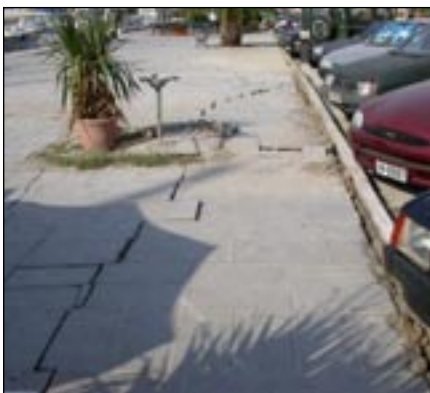
Figure 11. In the town of Lefkada, distorted pavement and sidewalks due to ground settlement and lateral spread (ITSAK team).
