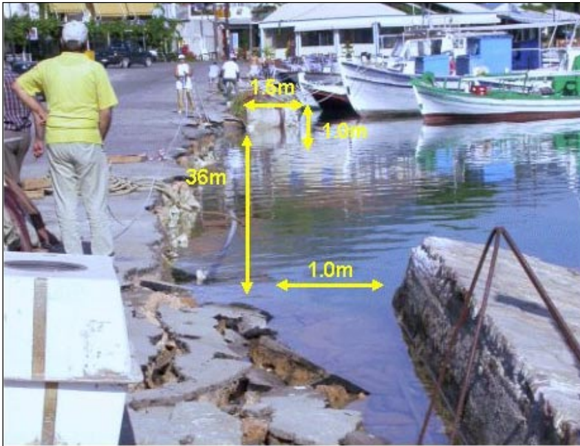
Figure 13. Part of the seawall has been laterally shifted and overturned (ITSAK team).
