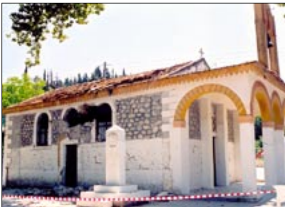
Figure 22. Churches built of stone masonry suffered heavy damage. In various parts of Lefkada, the tiles at the center of roofs moved. This might be explained by the vertical flexibility of the roof at its center (NTUA-UoA team).
