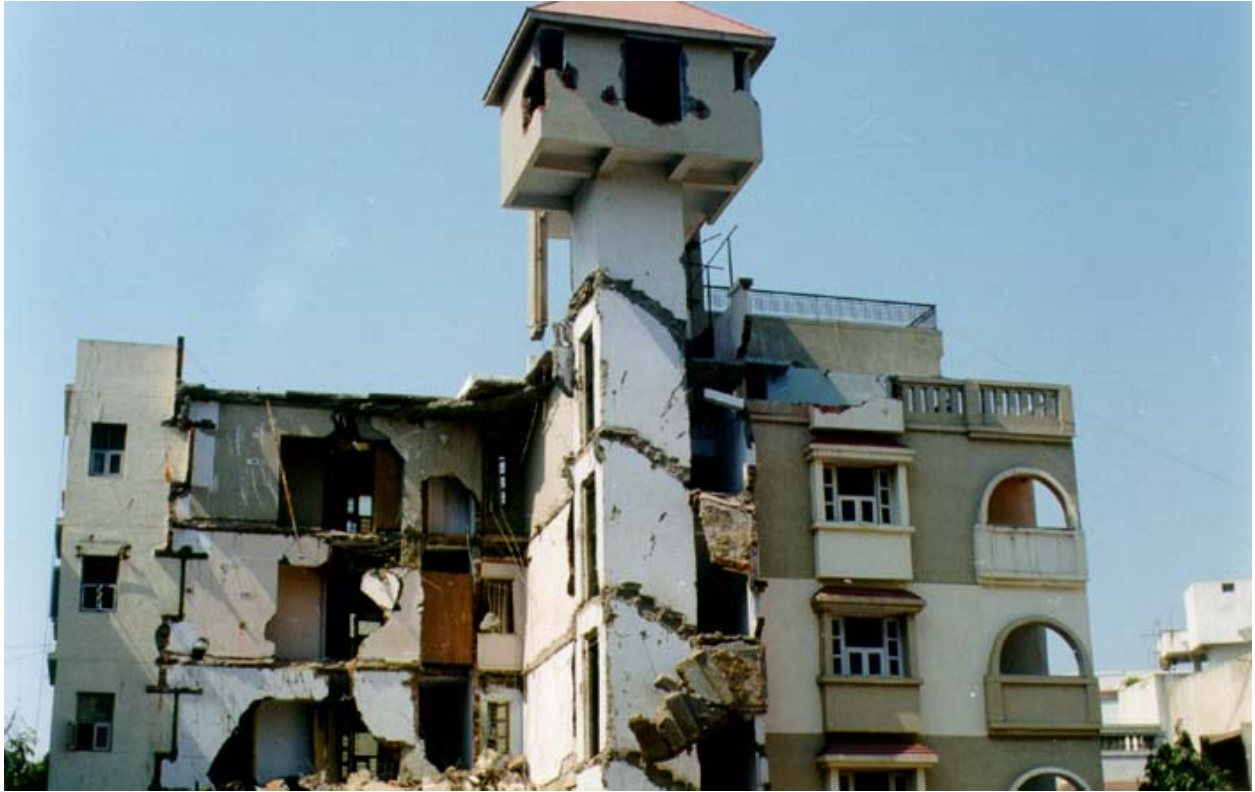
Figure 6I: Under-Utilization of Shear Capacity of Elevator Core Due to Improper Diaphragm Action of Slabs Resulted in Failure of an Apartment Building (2001 Bhuj Earthquake)
