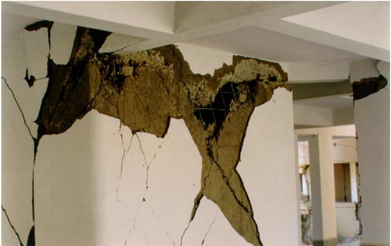
Figure 6K: View of Shear Damage of an Elevator Core (2001 Bhuj Earthquake)
