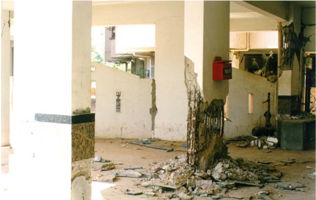
Figure 6C: Severe Damage and Plastic Hinging of Ground-Floor Column Due to Improper Confinement of Concrete and Lapping of Large Number of Longitudinal Bars
