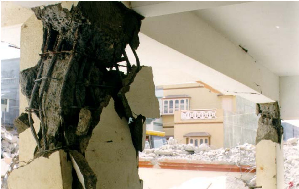
Figure 6J: Shear Failure of Column Just Below the Beam-Column Junction Due to Poor Construction
