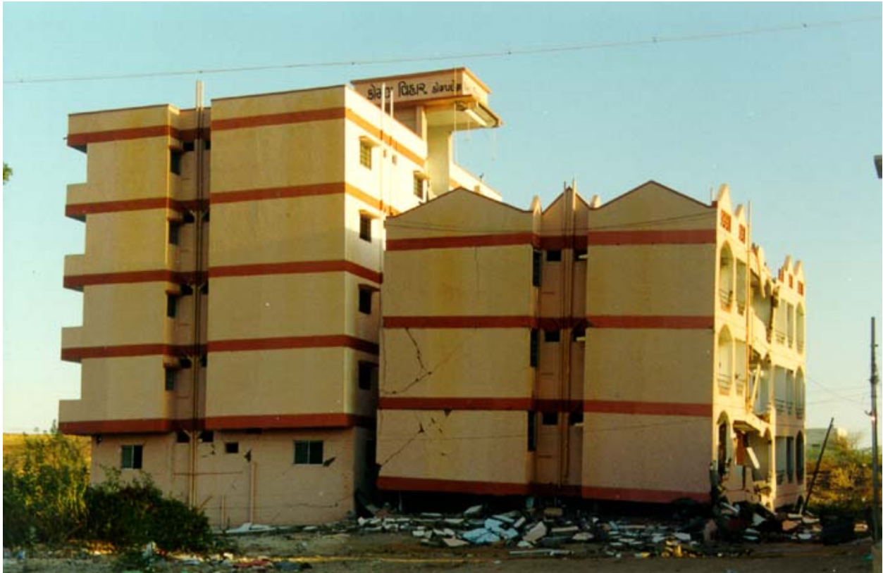
Figure 6H: Failure of Lower Two Stories of the Right Wing of an Apartment Building With Soft Storey; Note that the Left Wing Without Soft Storey is Apparently Undamaged (2001 Bhuj Earthquake)
