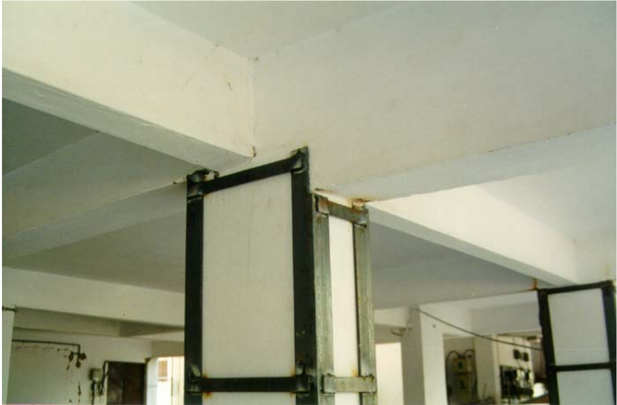
Figure 7D: Termination of Column Jacket Steel at Beam Soffit Level Resulting in No Increase in Moment Capacity of Column (2001 Bhuj Earthquake)
