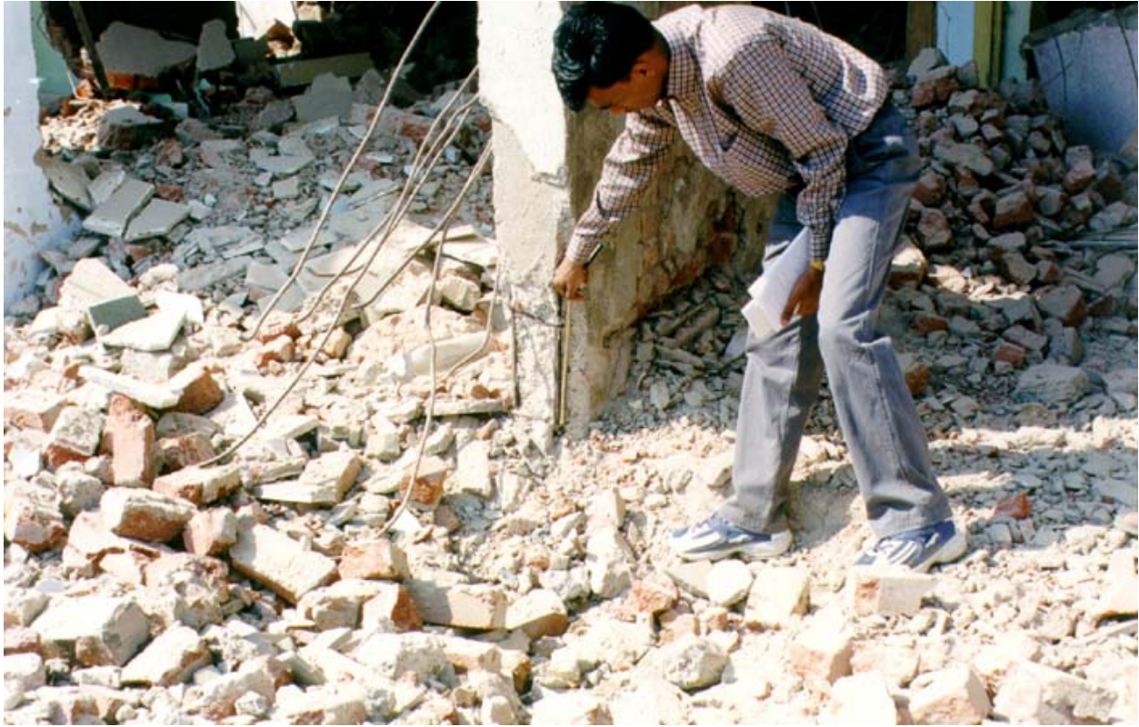
Figure 6E: Damage to Ground Floor Columns Due to Inadequate Lateral Confinement of Reinforcement Bars
