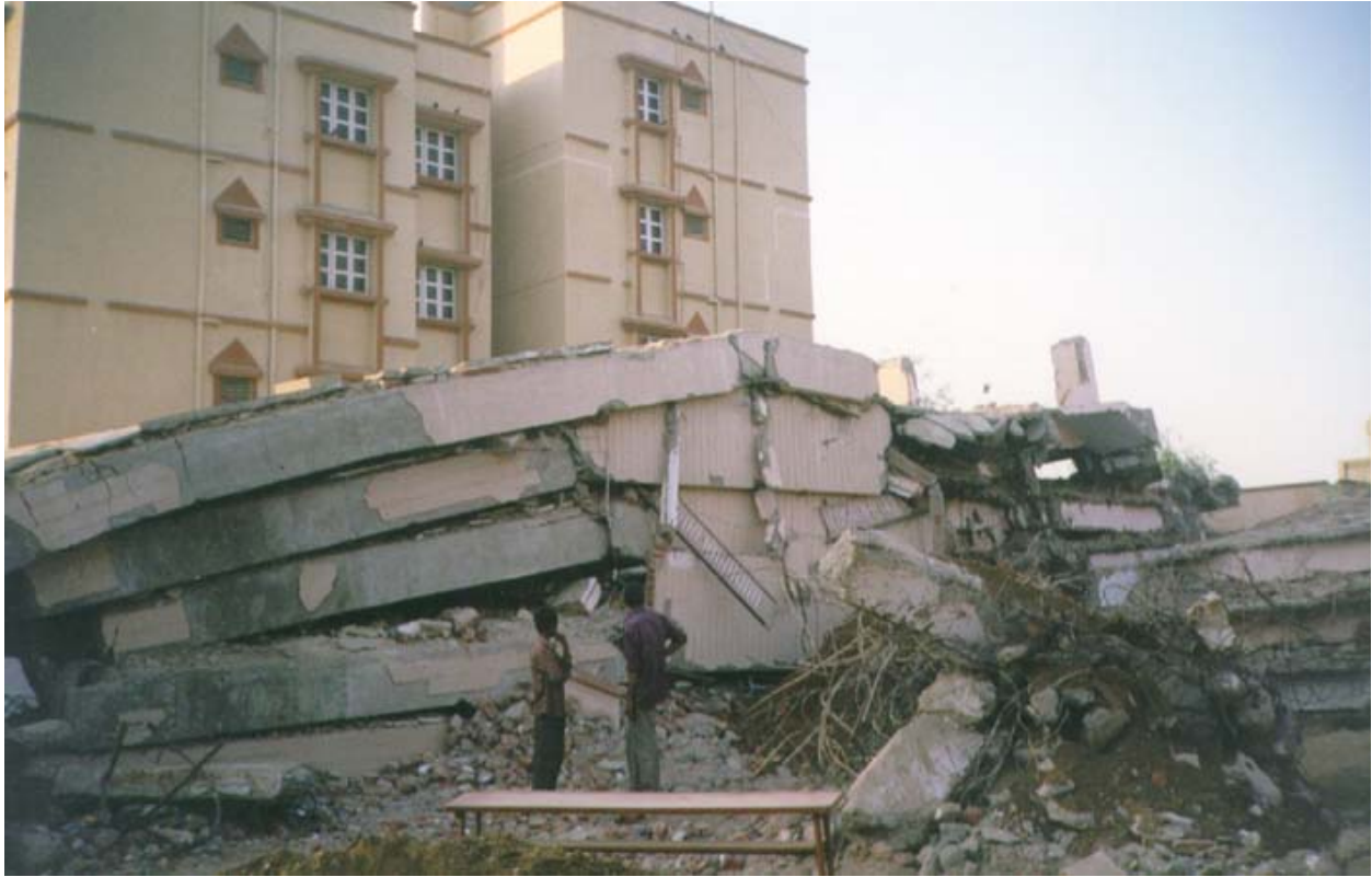
Figure 6L: Pancake Collapse of a Multi-Storey Building Due to Weak Column-Strong Beam Design (2001 Bhuj Earthquake)
