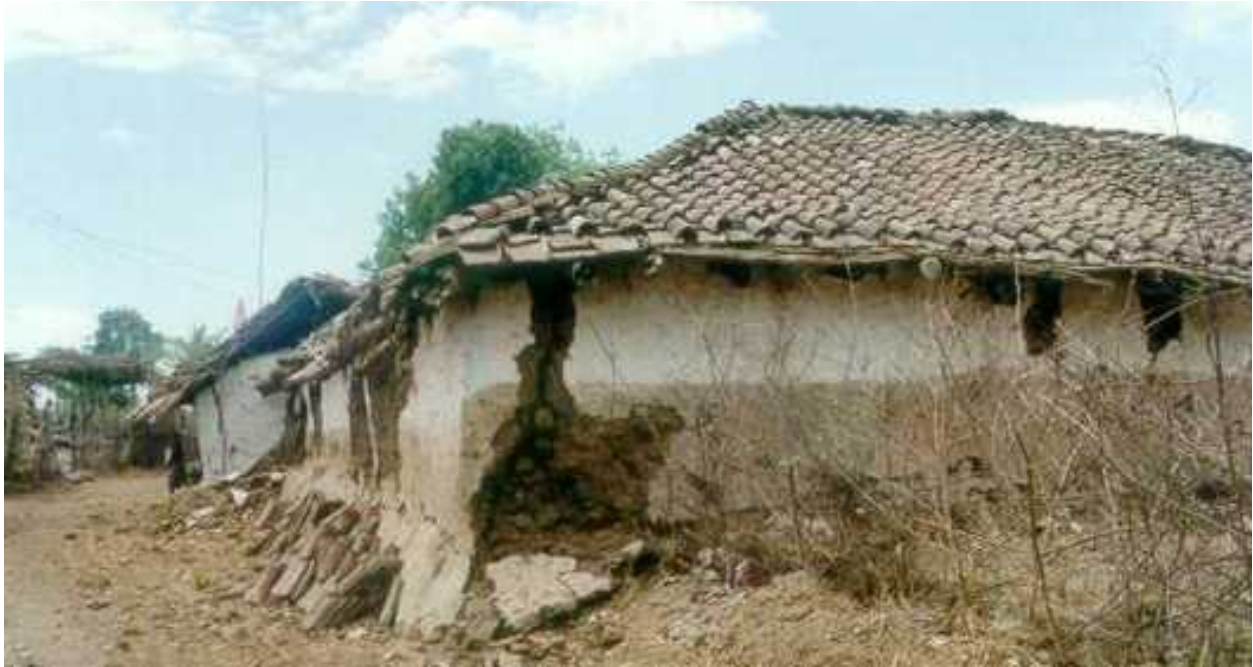
FIGURE 6C: Typical Earthquake Damage - Crushing of Mud Walls in the 1997 Jabalpur earthquake (Source: Sudhir K. Jain, IIT Kanpur)
