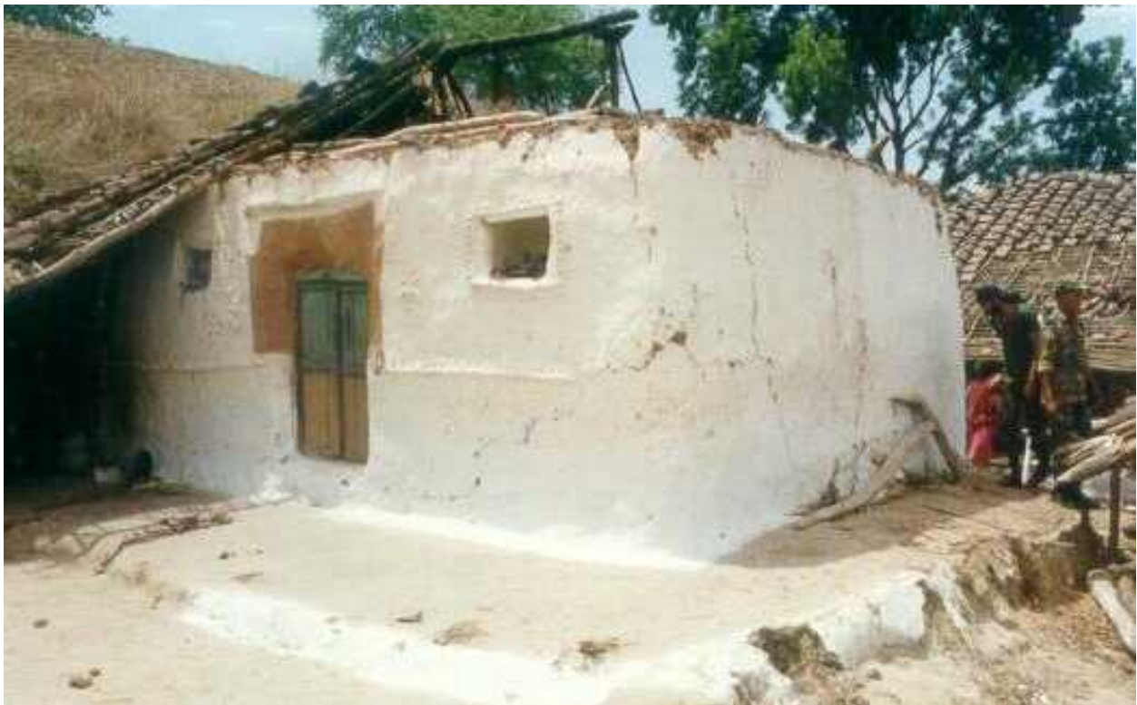
FIGURE 6D: Typical Earthquake Damage - Roof Collapse in the 1997 Jabalpur earthquake (Source: Sudhir K. Jain, IIT Kanpur)
