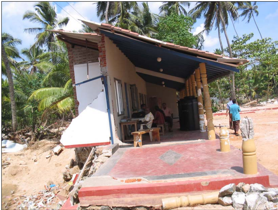
Figure 3. Damaged housing, south of Relief Camp Peraliya, Sri Lanka (photo: Tricia Wachtendorf).
