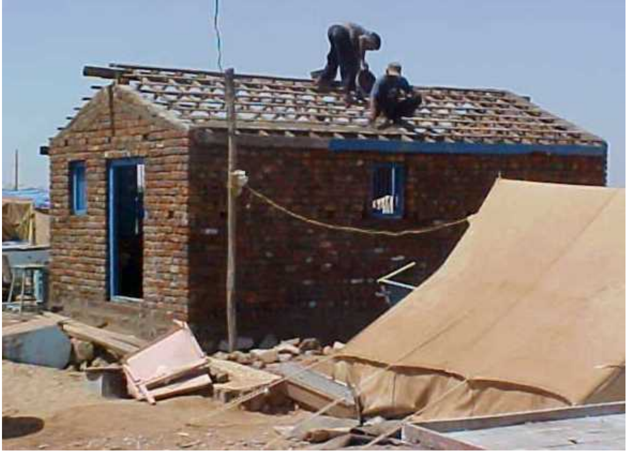
FIGURE 2B: Key Load-Bearing Elements - Roof Construction (Source: Sudhir K. Jain, IIT Kanpur)
