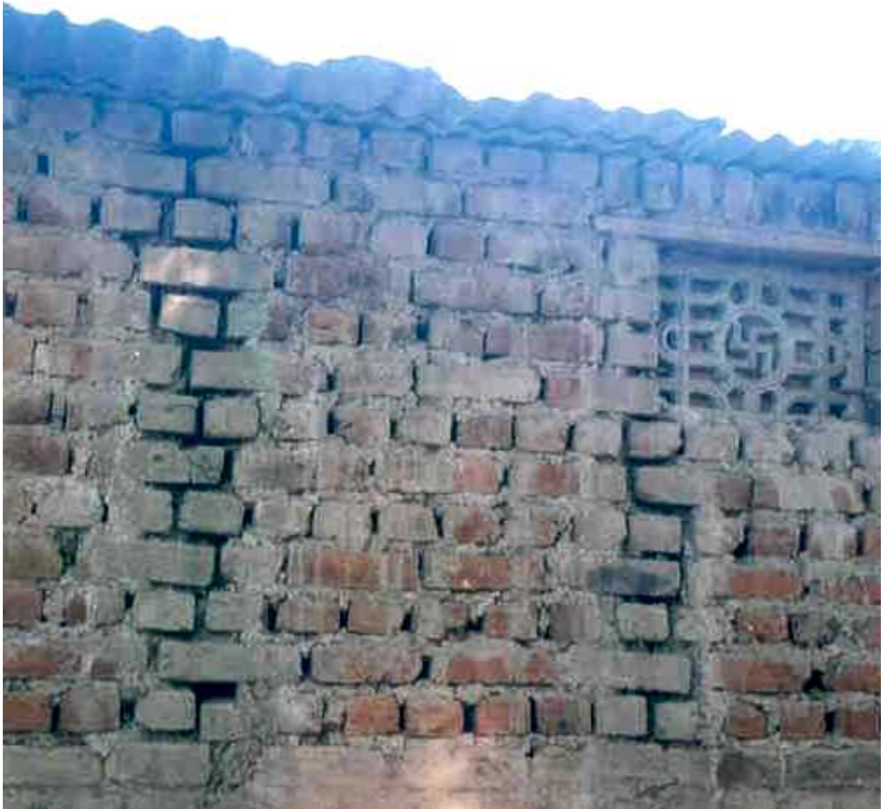
FIGURE 4: Critical Structural Details - Elevation of Brick Masonry Wall in Mud Mortar (Source: Svetlana Brzev)
