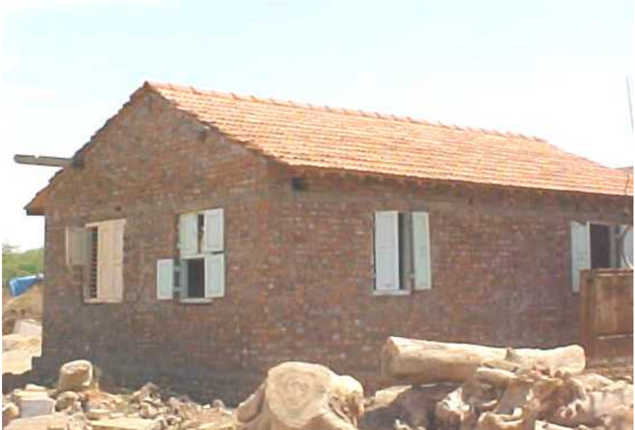
FIGURE 5A: Key Seismic Resilient Features - RC Lintel Band and Good Quality Brick Masonry Construction (Source: Sudhir K. Jain, IIT Kanpur)
