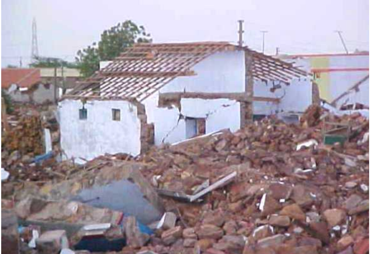
FIGURE 6C: Typical Earthquake Damage: Collapse of roof and walls of a brick lime mortar house in the 2001 Bhuj earthquake (Source: Sudhir K. Jain, IIT Kanpur)
