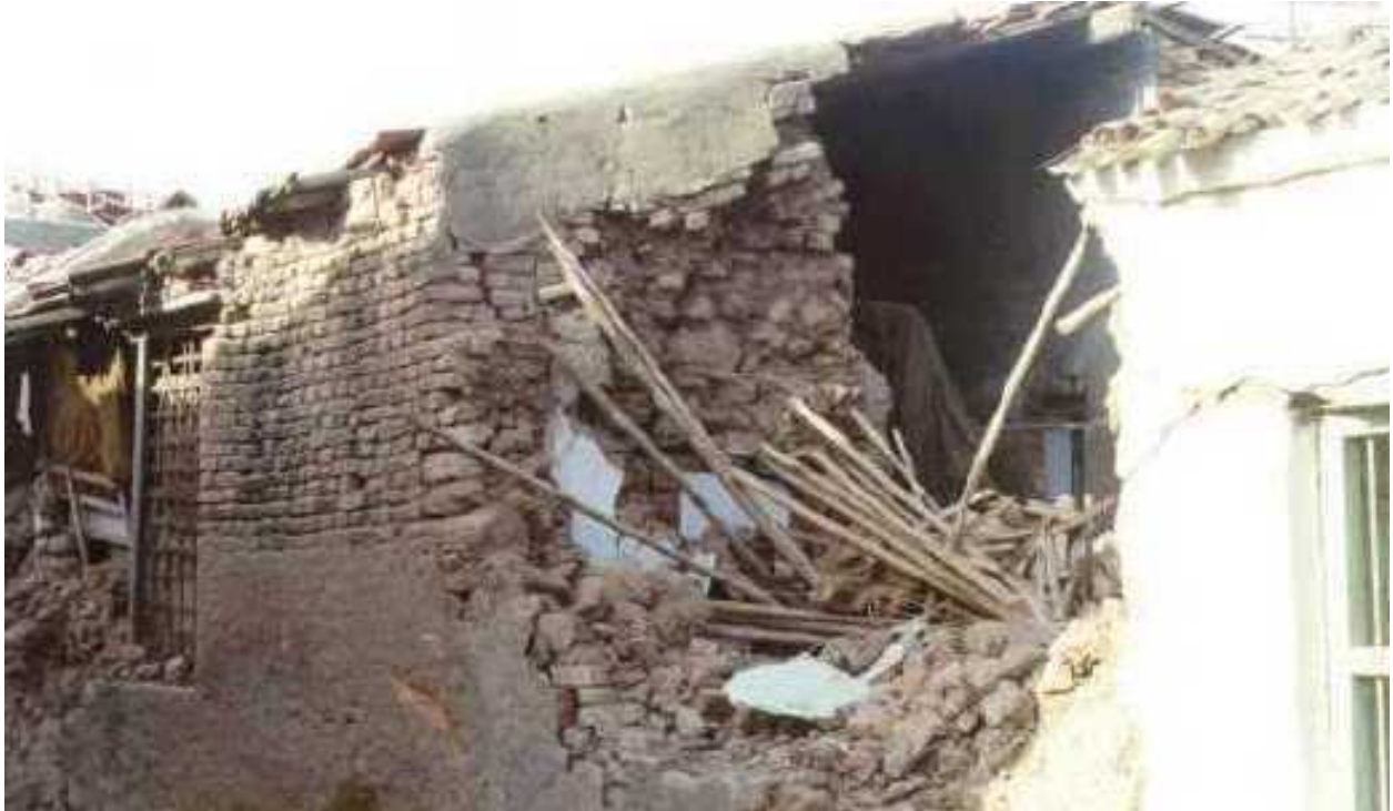
FIGURE 6A: Typical Earthquake Damage - Wall Collapse due to Poor Quality Brick Construction and Poor Inadequate Wall Connections in the 2001 Bhuj earthquake (Source: IIT Powai 2001)
