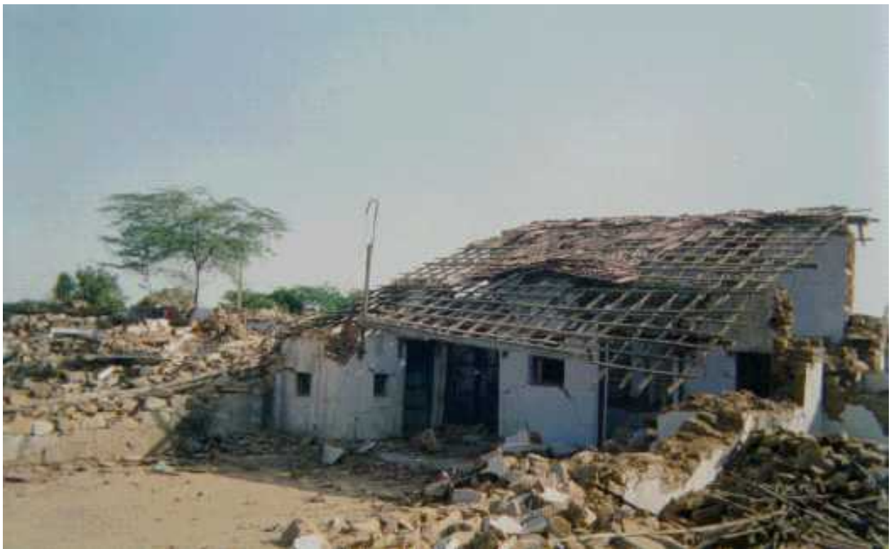
FIGURE 6B: Failure of a residential building, Chobri Village near Bhachau, 2001 Bhuj earthquake (Source: IIT Powai 2001)
