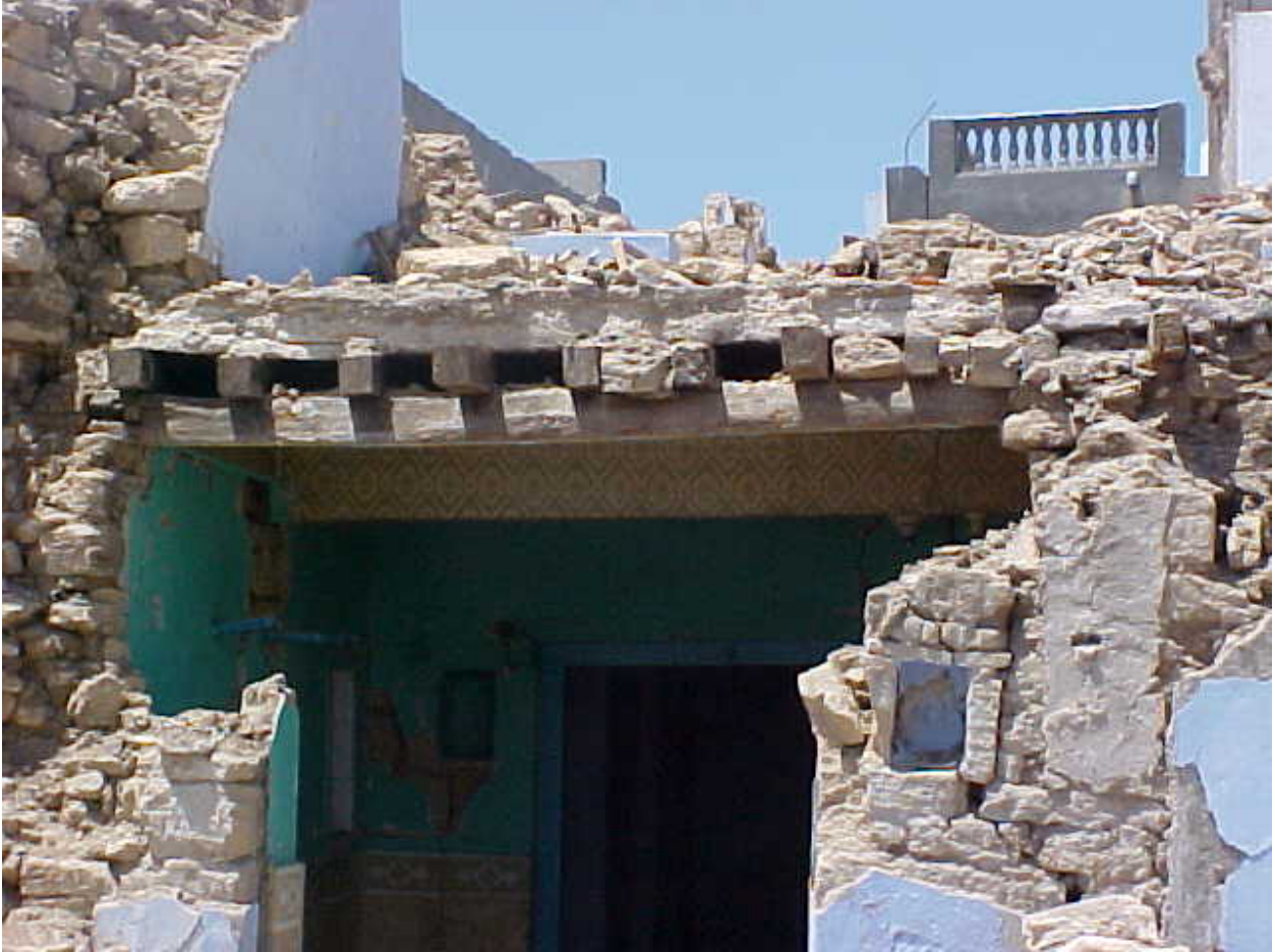
FIGURE 6: Typical Earthquake Damage in the 2001 Bhuj earthquake (Source: Sudhir K. Jain, IIT Kanpur)
