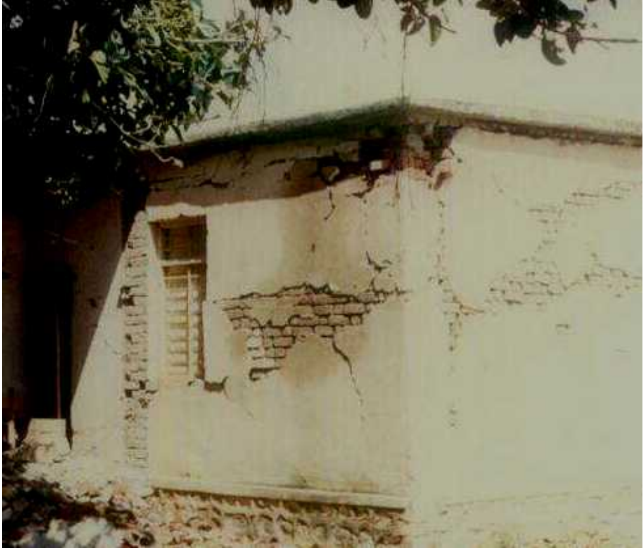
FIGURE 4B: Critical Structural Details - Unreinforced Brick Masonry Wall in Mud Mortar (1993 Killari Earthquake), Source: Sudhir K. Jain, IIT Kanpur
