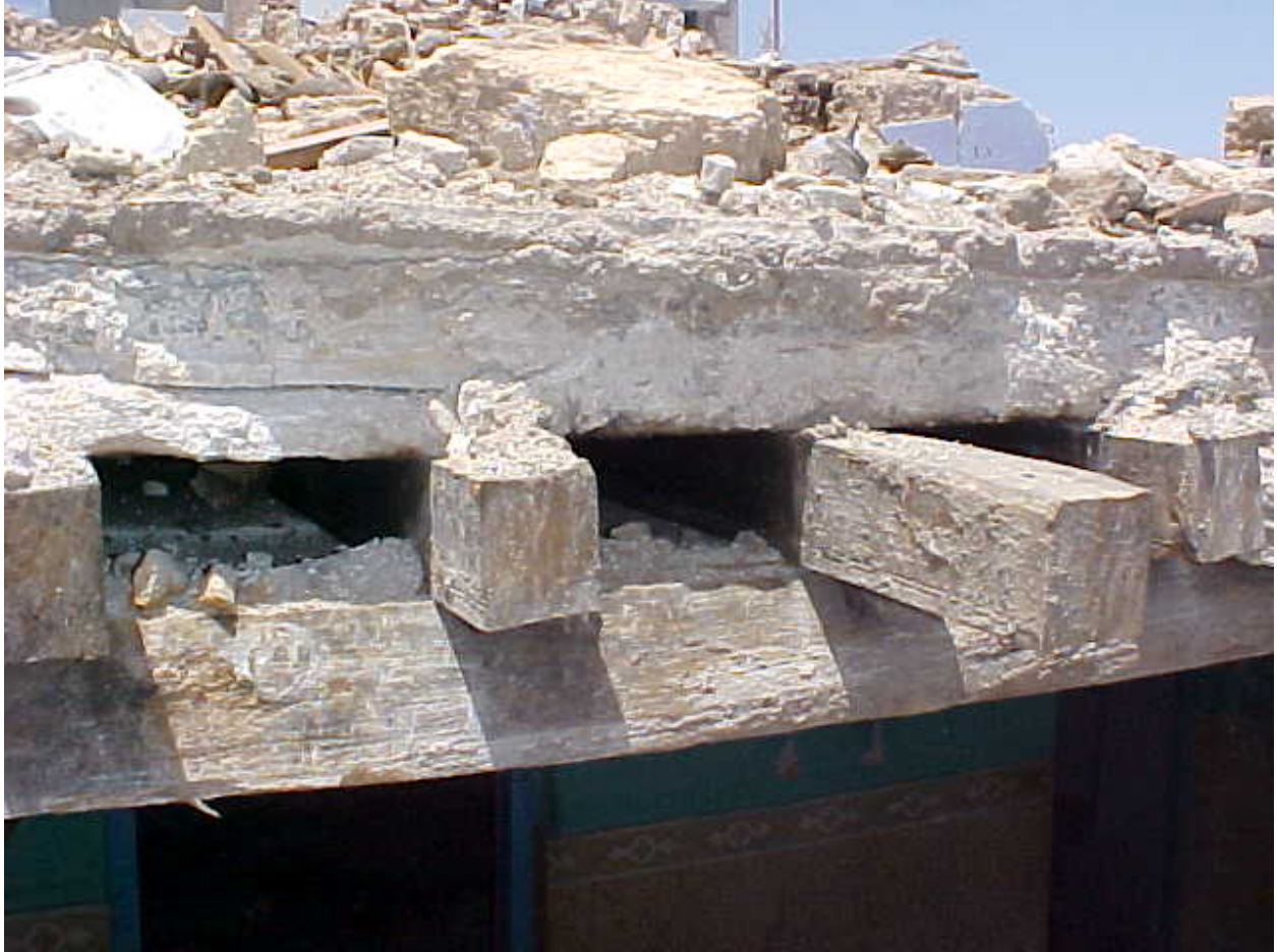
FIGURE 5: Key Seismic Deficiencies - Heavy Roof
