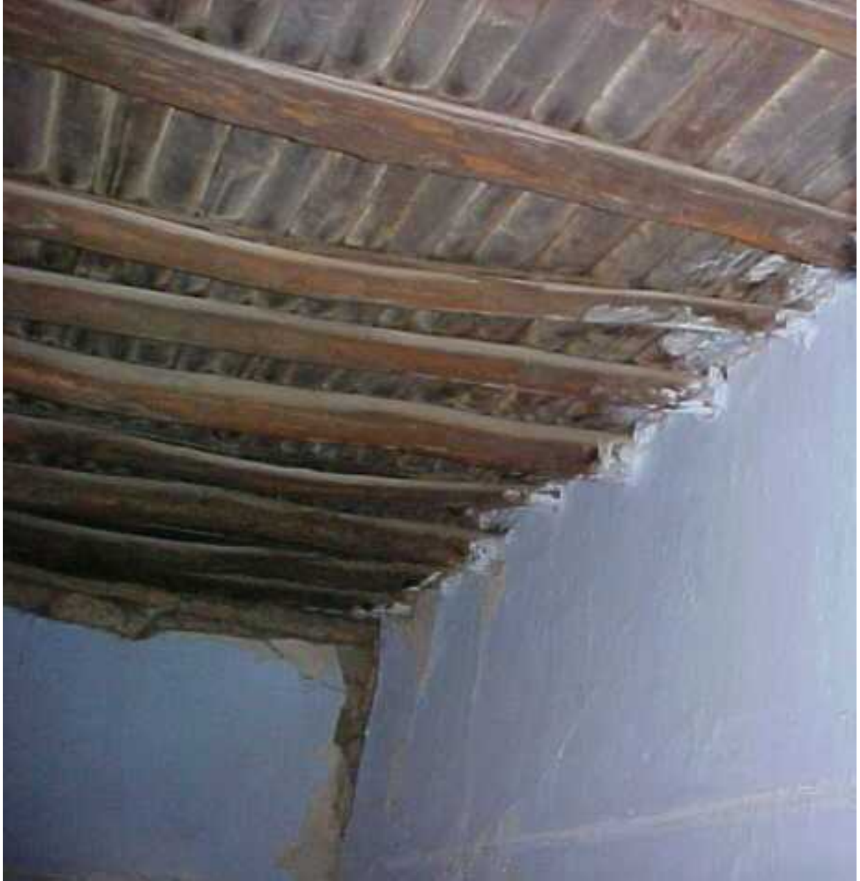
FIGURE 4A: Critical Structural Details - Roof Structure (Source: Sudhir K. Jain, IIT Kanpur)
