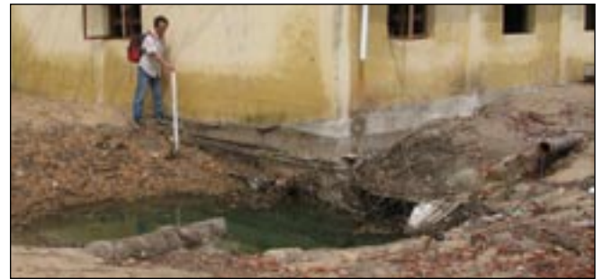
Figure 5. Tsunami scour and failure of a wastewater pipe at a schoolhouse at Kalapakkom.
