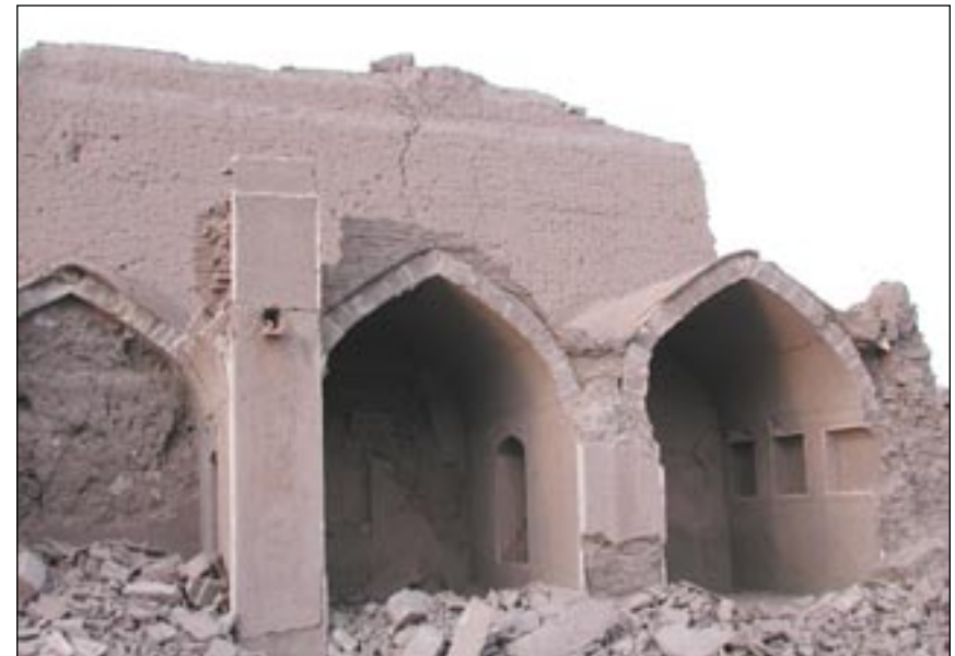
Figure 14 Out-of-plane collapse of adobe walls in Arge-Bam.
