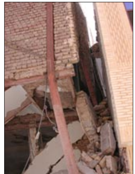
Figure 20 Typical weak-story collapse.
