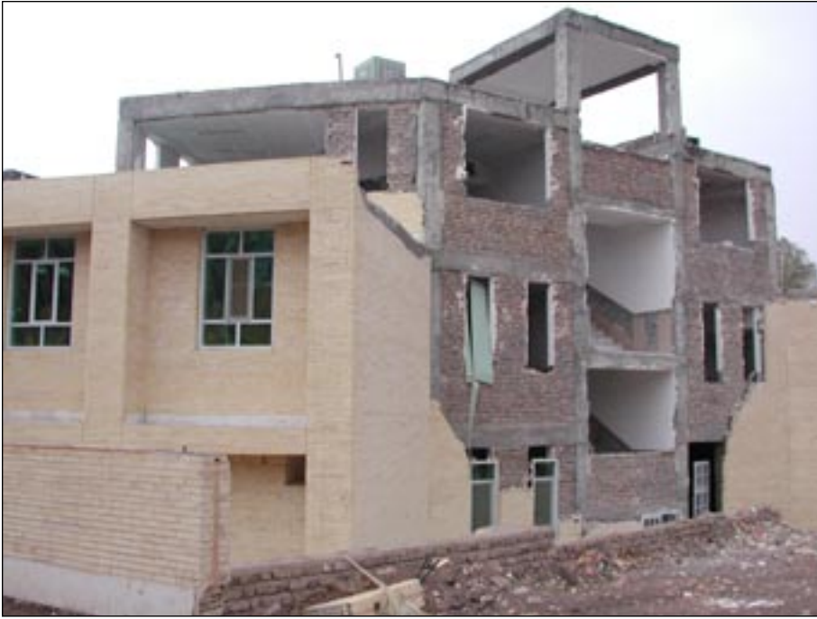
Figure 21 Substantial damage to a hospital building.
