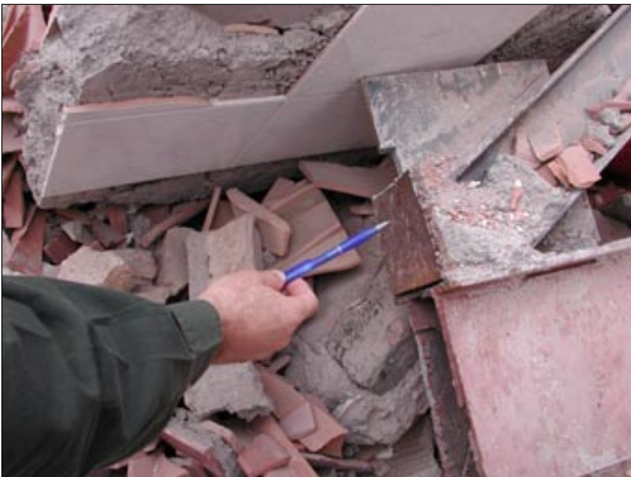
Figure 19 Collapse of steel-framed dual-system building at least partially due to deficient welding practice.
