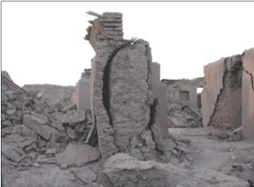
Figure 15 Addition of exterior layers to the core adobe walls suggests earlier repair of earthquake damage.
