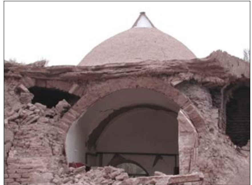
Figure 16 Failure of large adobe house.
