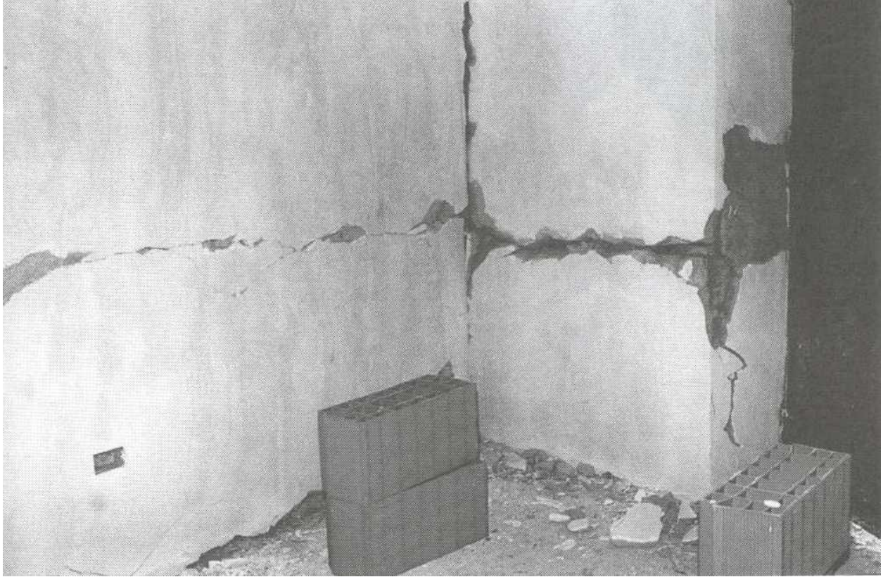
FIGURE 7G: Seismic Strengthening - Damage of Wall Strengthened by Shotcreting
