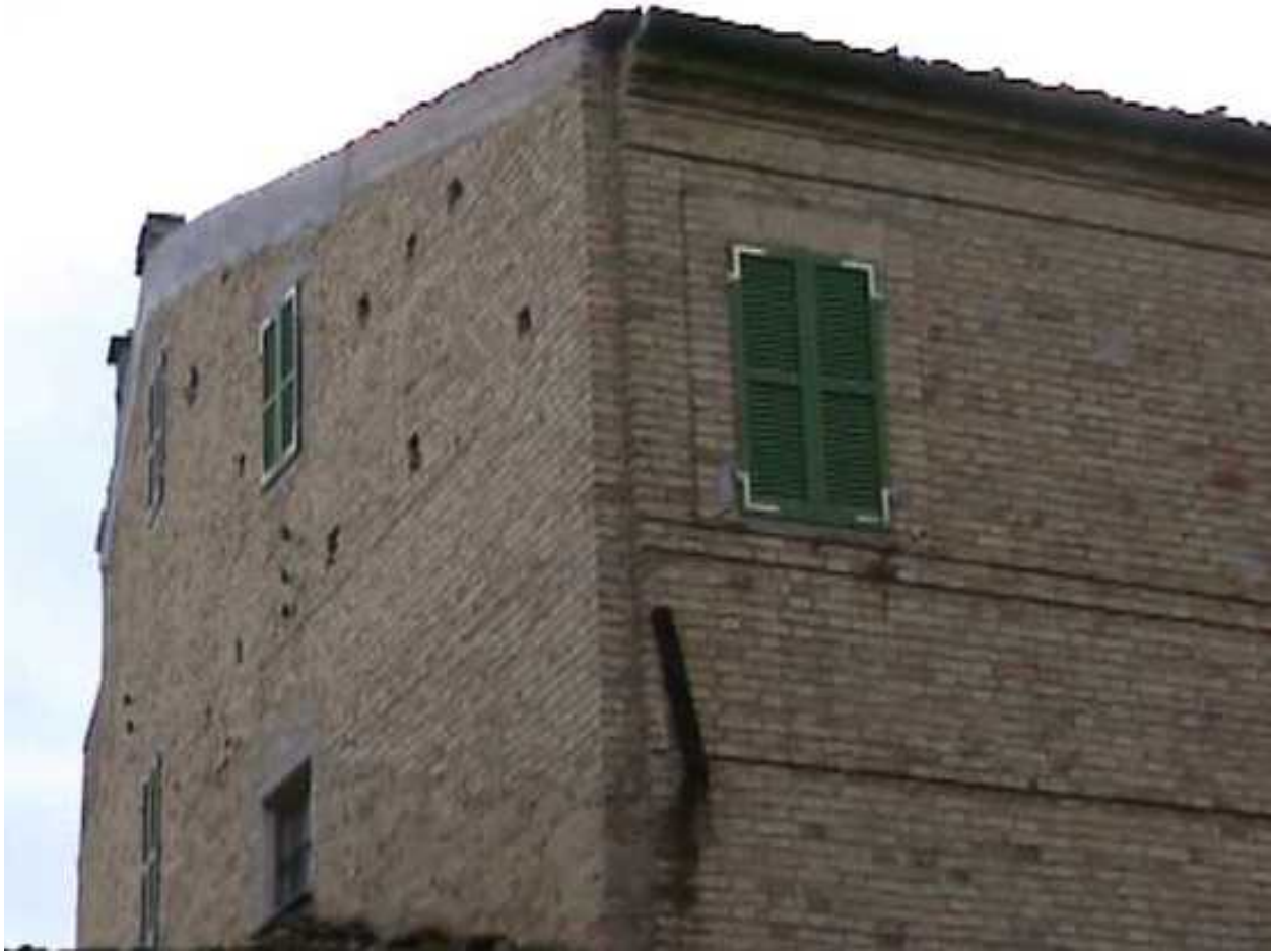
FIGURE 7C: Seismic Strengthening - Installation of a New RC Ring Beam at the Roof Level (Design Application)
