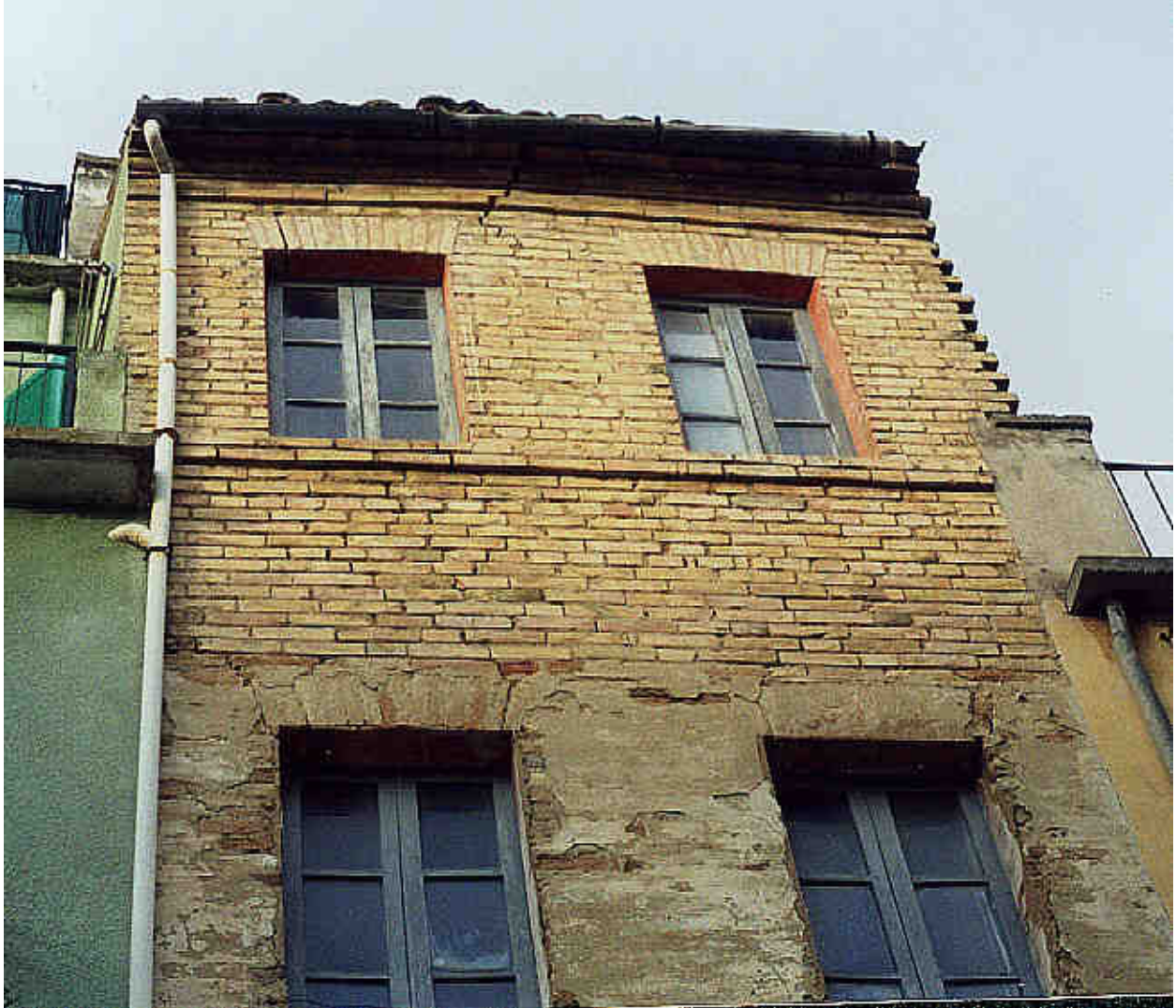
FIGURE 6: A Photograph Illustrating Typical Earthquake Damage (1997 Umbria-Marche earthquake)
