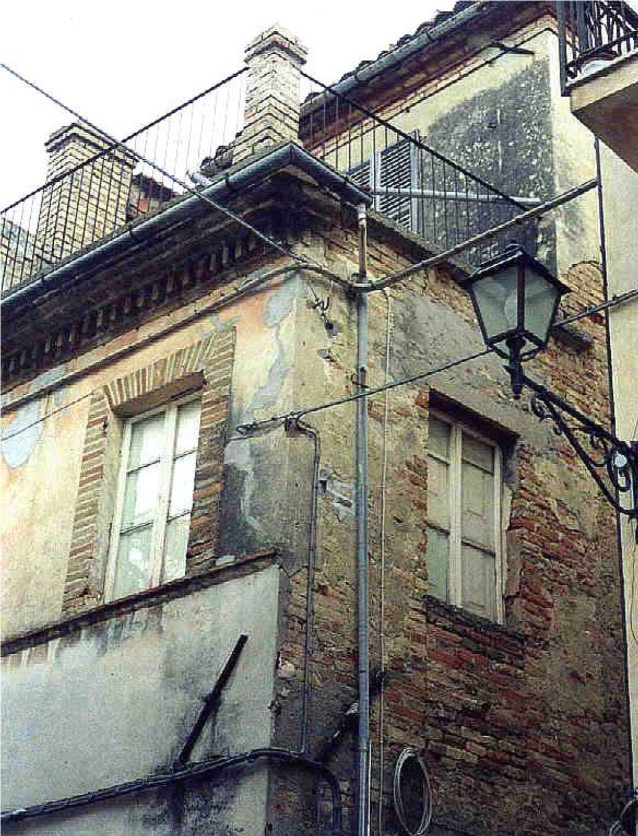
FIGURE 5A: Key Seismic Deficiencies-Proximity of Windows to the Corners and Vertical Extension of the Building (note also added balconies)
