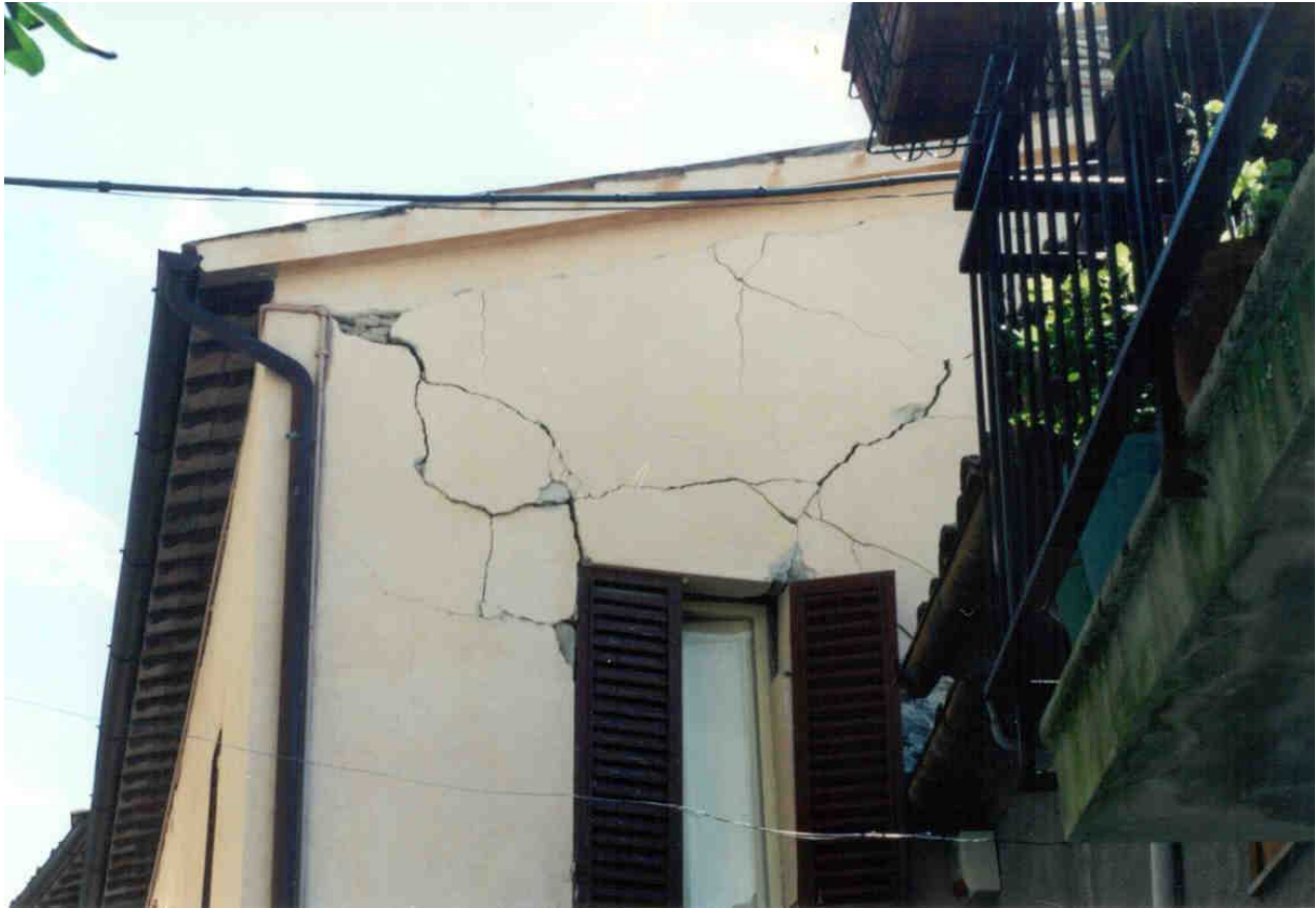
FIGURE 6B: Earthquake Damage to a Retrofitted Building Due to the Inadequate RC Ring Beam-Wall Connection
