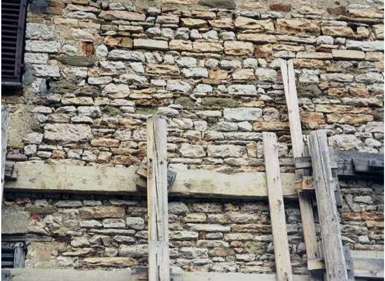
FIGURE 4A: Critical Structural Details Stone Masonry Wall With Irregular Roughly Dressed Stone Blocks of Varying Dimensions Embedded into Thick Lime Mortar Joints (not properly repointed)
