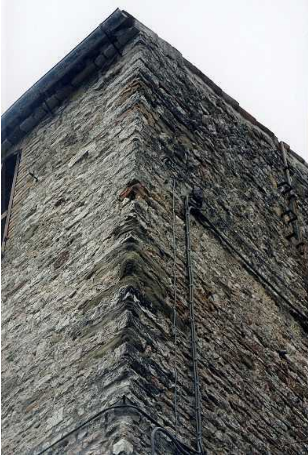
FIGURE 5B: Earthquake-Resilient Feature - Corner Returns between the Perpendicular Walls Made of Larger Stone Blocks
