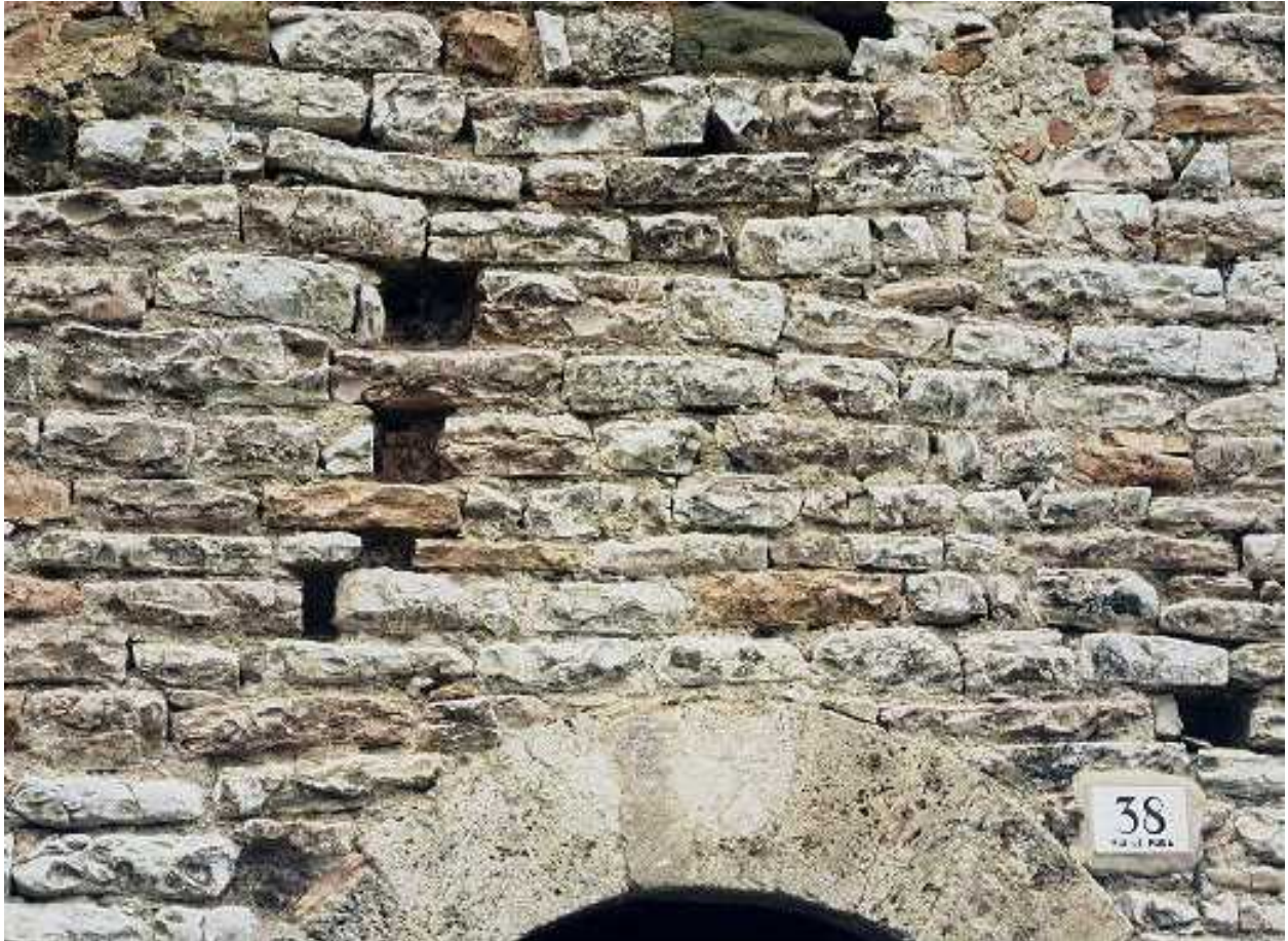
FIGURE 4B: Critical Structural Details-Movement Between the Blocks, Probably as a Result of Damage in Previous Earthquakes and Visible Loose Stones Around the Arch
