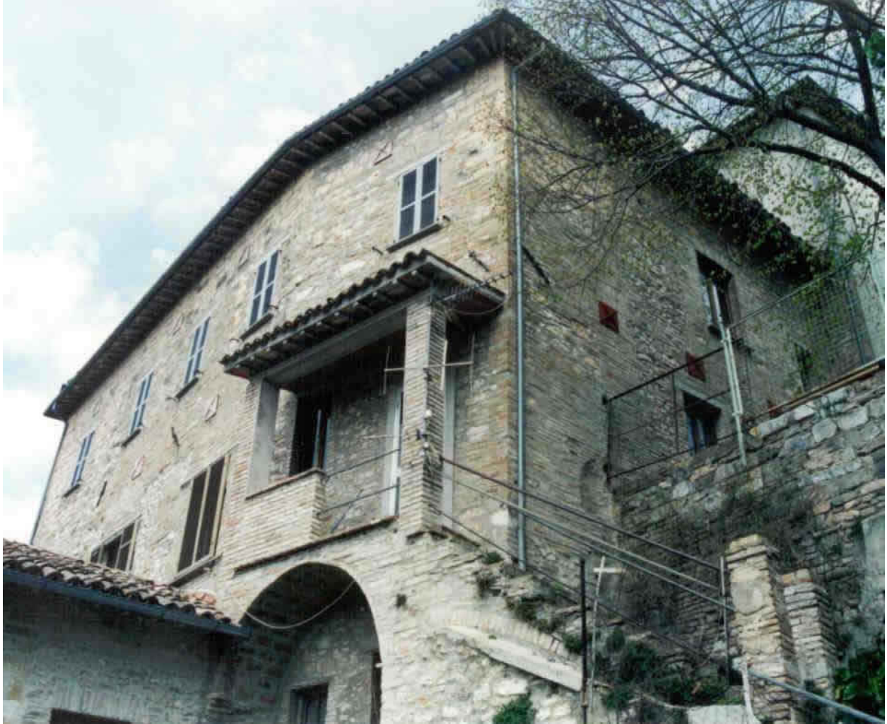
FIGURE 7B: Seismic Strengthening Techniques- Installation of modern anchors with anchorage plates and concrete lintels over openings
