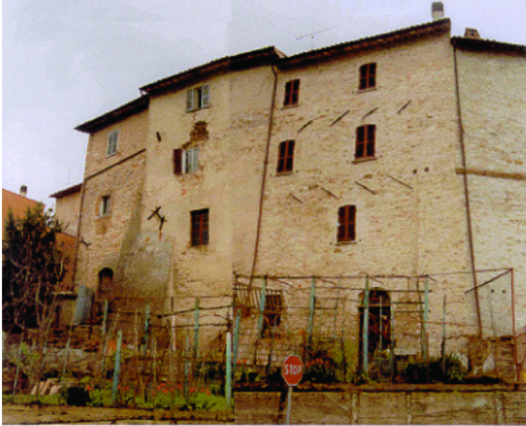
FIGURE 5A: Key Seismic Features and Deficiencies Showing the Regular Arrays of Floor Ties in One Unit, Irregular Distribution of Wall Ties in the Next One, and Corner Return Stones in the Third Unit.
