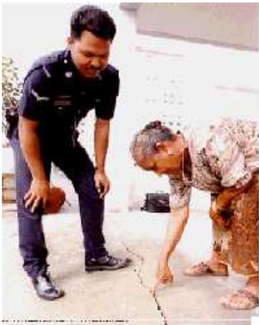
FIGURE 5B: Typical Earthquake Damage (Penang (M6.0) earthquake of 10 October 1996)
