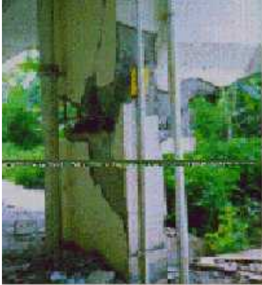
FIGURE 5A: A Photograph Illustrating Typical Earthquake Damage in the Labuan, Sabah (M5.8) of 26 May 1991
