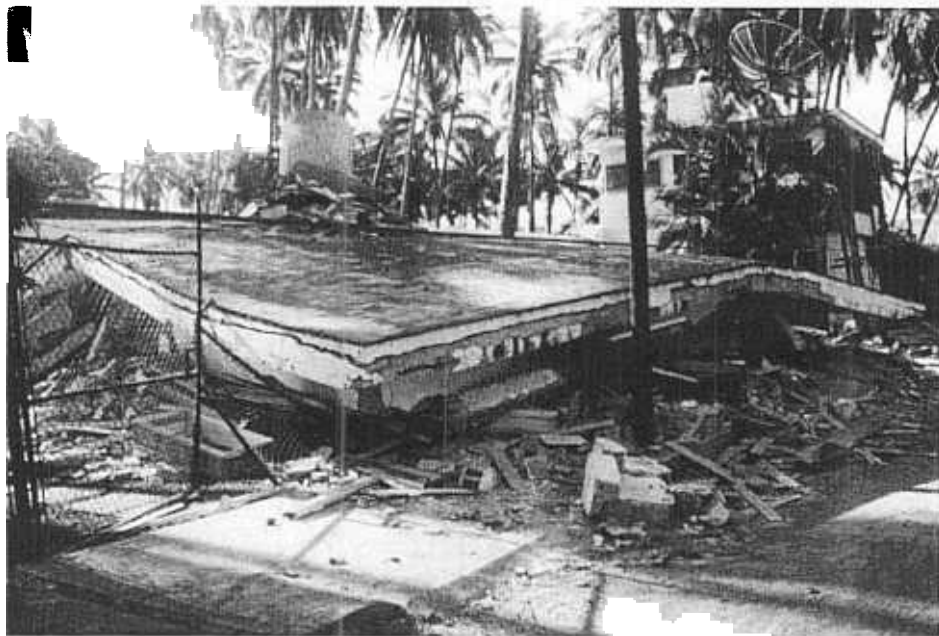
Figure 4 - This two-story home in Manzanillo collapsed due to a heavy roof and inadequate walls.
