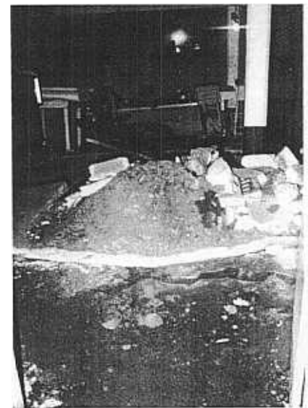
Figure 1 - Liquefaction caused a sand boil that forced its way through the weak concrete foundation of this home.
