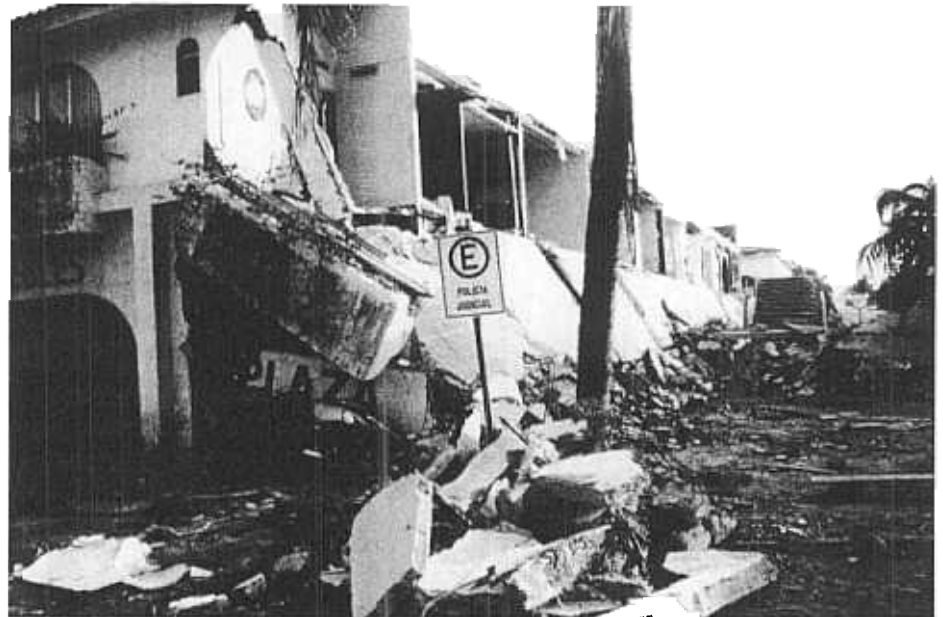
Figure 3 - The partial collapse of a two-story office building in a Santiago shopping center was due to inadequate exterior columns.
