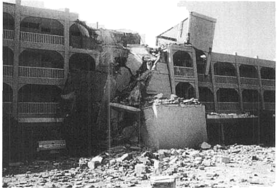
Figure 2 - A collapsed stair tower at the Casa Grande Resort in Melaque. A 45-ton water tank constructed on top of the stair tower probably contributed to its failure.
