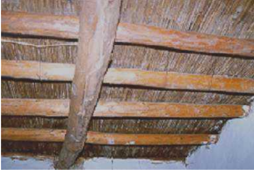
FIGURE 5A: Seismic Deficiencies - Inadequate Wall-Roof Connections
