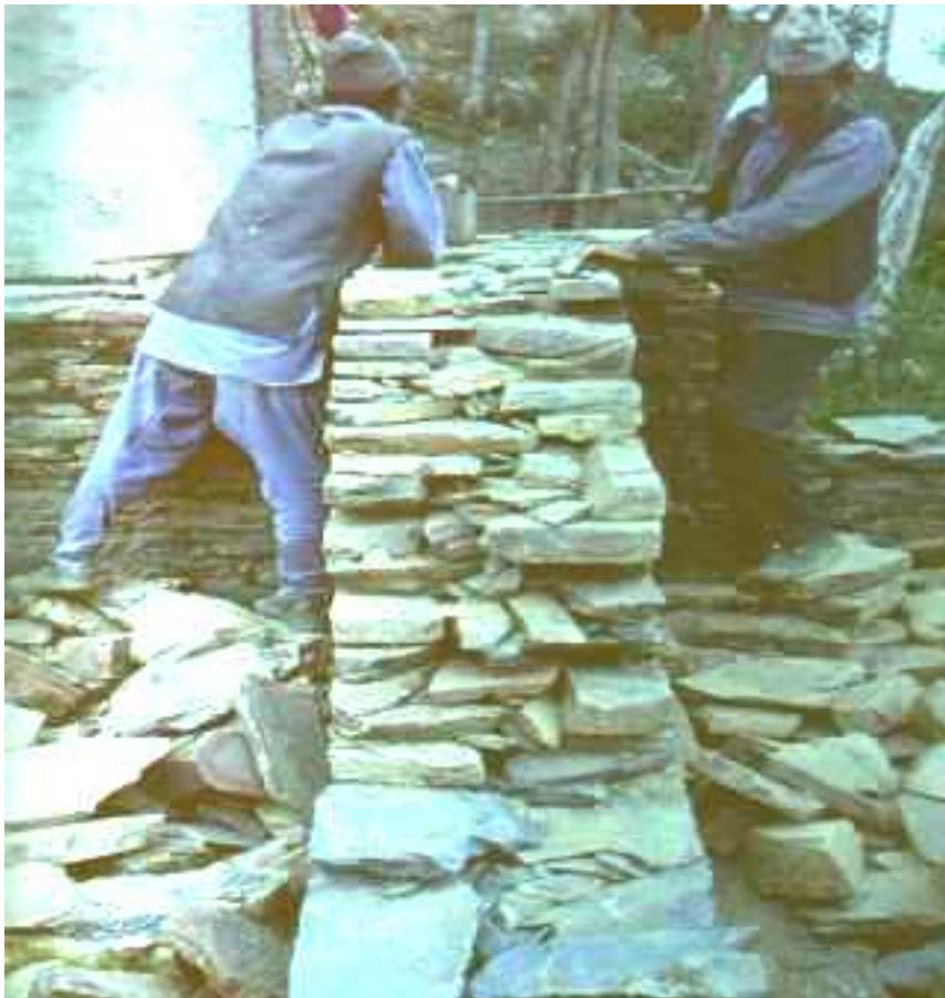
FIGURE 5: Key Seismic Deficiencies-Lack of Connection Between the Wall Wythes (note loose stone rubble)
