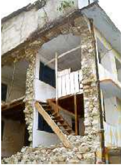
FIGURE 6D: Typical Earthquake Damage -Out-of-plane Wall Collapse Due to Lack of Anchorage
