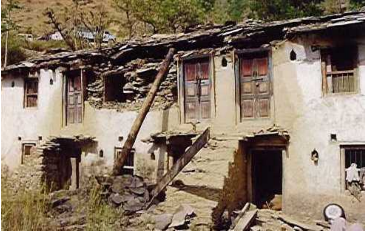
FIGURE 6B: Typical Earthquake Damage to Stone Masonry Buildings
