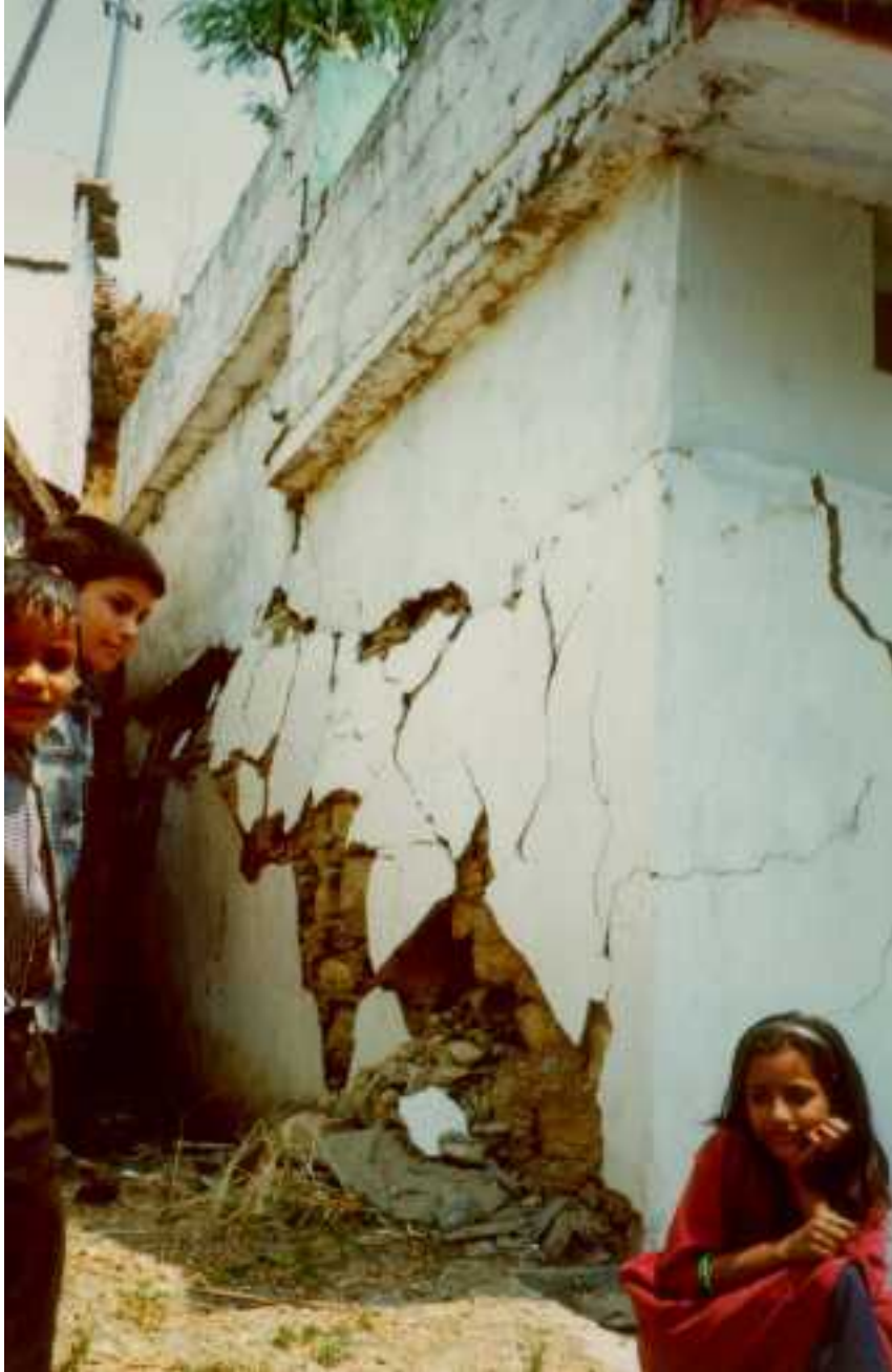
FIGURE 6E: Typical Earthquake Damage -Wall Bulging due to Delamination
