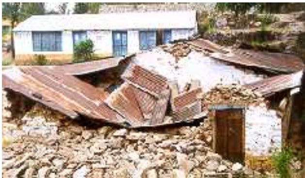
FIGURE 6C: Complete Collapse of a Stone Building in an Earthquake
