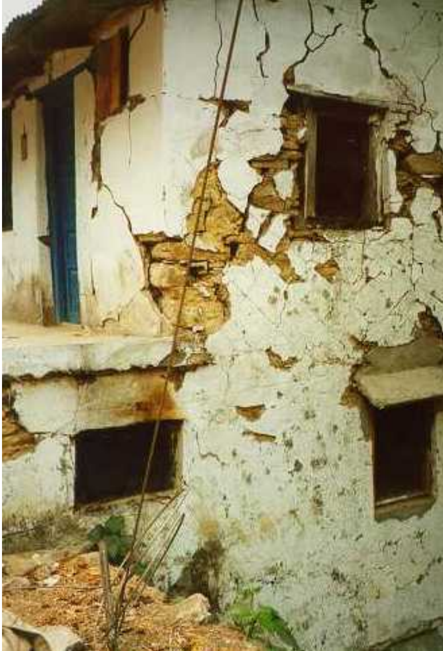
FIGURE 6F: Typical Earthquake Damage - In-plane Failure of a Stone Masonry Wall
