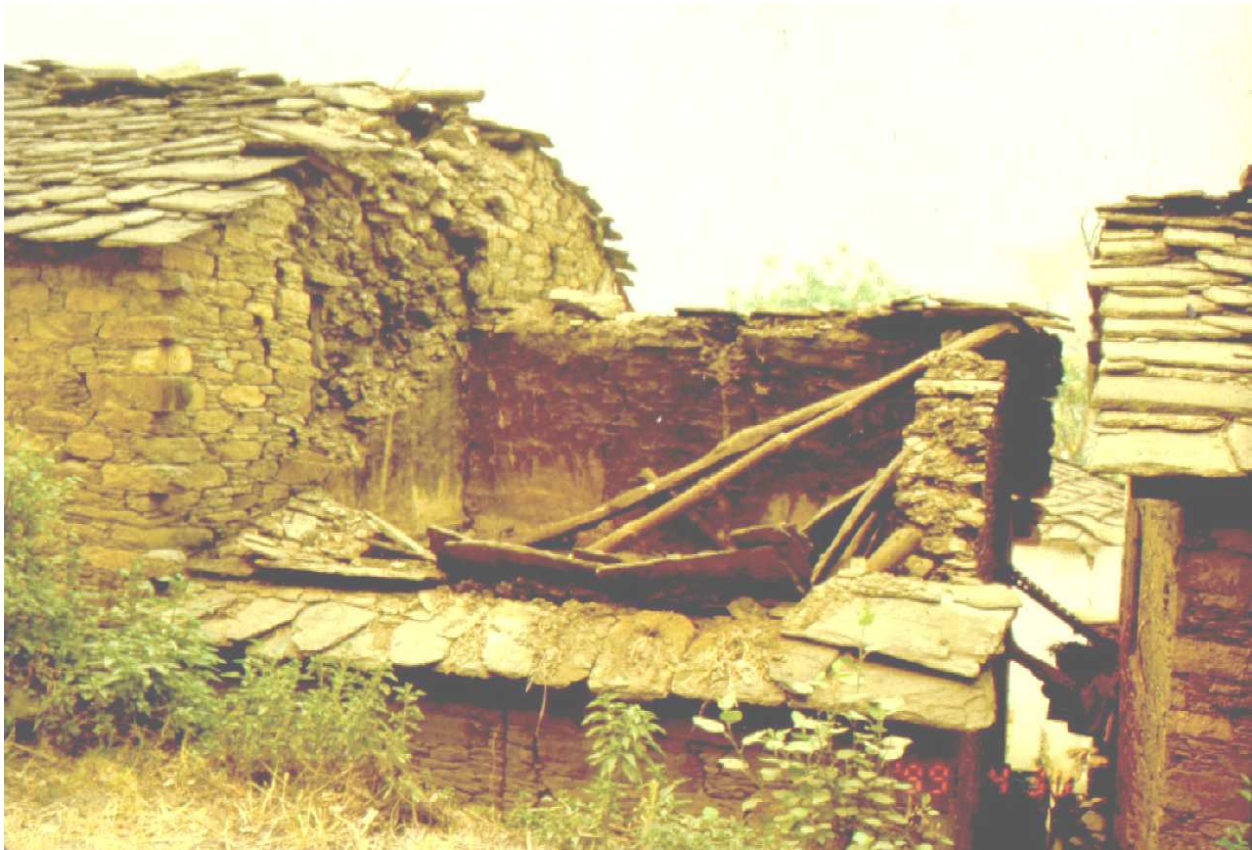
FIGURE 6: Typical Earthquake Damage-Roof Collapse Due to the Absence of Wall-Roof Connection
