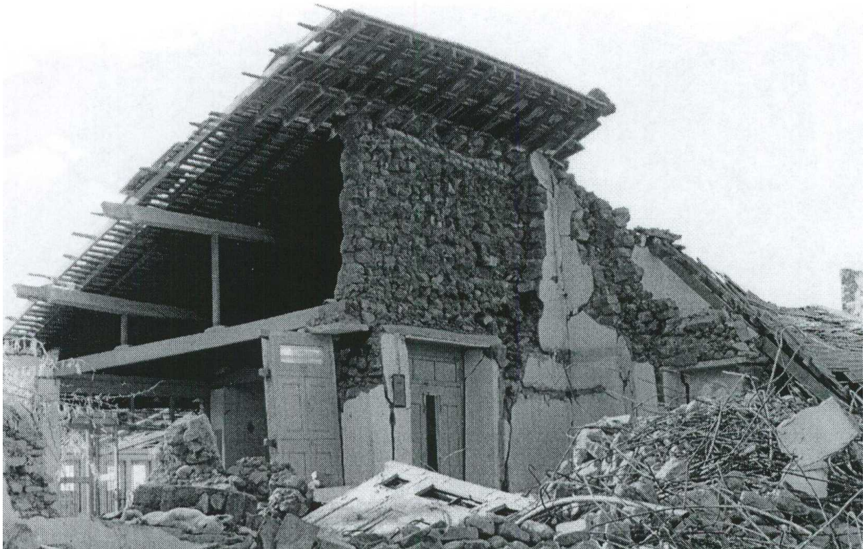
FIGURE 6A: Typical Earthquake Damage - Delamination of Stone Walls due to Absence of Bond Stones (through-stones)
