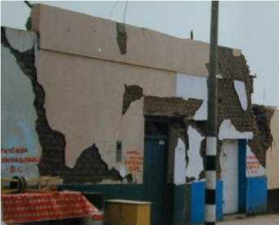
FIGURE 5B: Key Seismic Deficiencies - Wall Damage Due to Inadequate In-Plane Seismic Resistance
