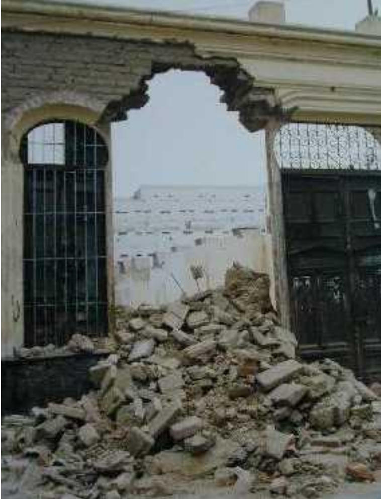
FIGURE 6A: A Photograph Illustrating Typical Earthquake Damage (November 1996 Nasca Earthquake)
