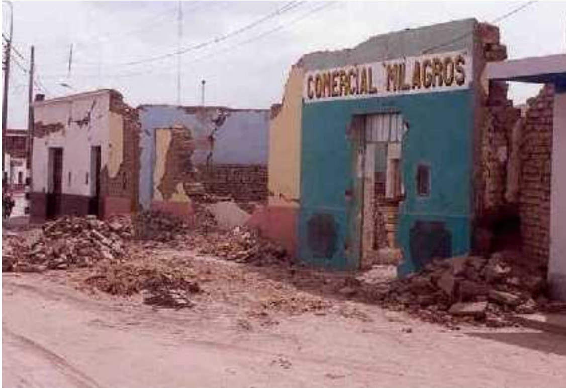
FIGURE 6B: A Photograph Illustrating Typical Earthquake Damage (November 1996 Nasca Earthquake)
