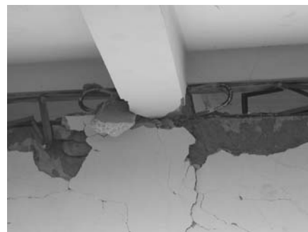
Figure 10 View of the collapse of one of the short columns in the school building shown in Figure 9. (Photo: E. Fierro)
