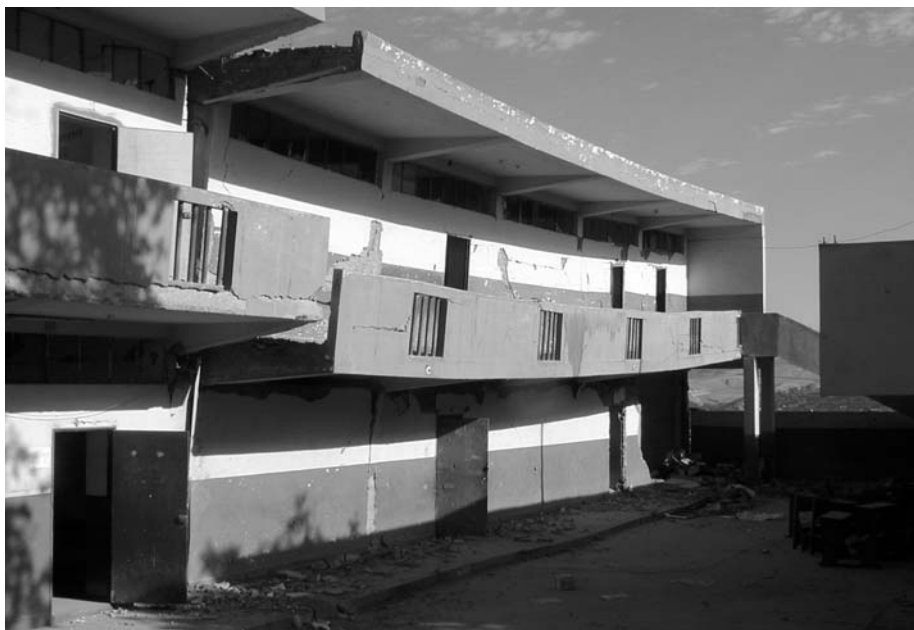
Figure 9 School building in Moquegua. Partial collapse due to failure of short columns. (Photo: E. Fierro)
