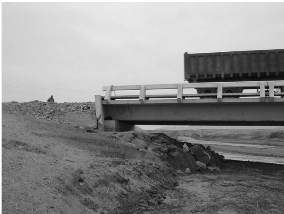
Figure 14 Damaged bridge abutment. (photo: Yashinsky)
