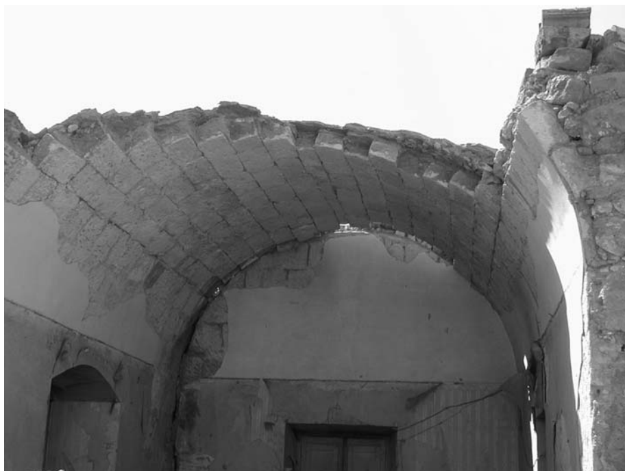
Figure 12 Damage to typical historic dwelling with vaulted roof constructed of "sillar" blocks. (Photo: E. Fierro)
