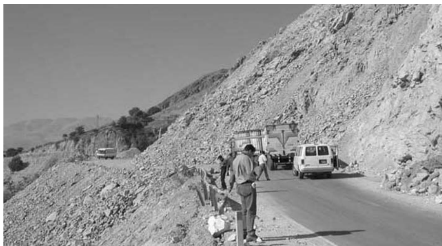
Figure 5 Slope failure along highway between Cuajone and Moquegua. (photo: geotechnical reconnaissance team)
