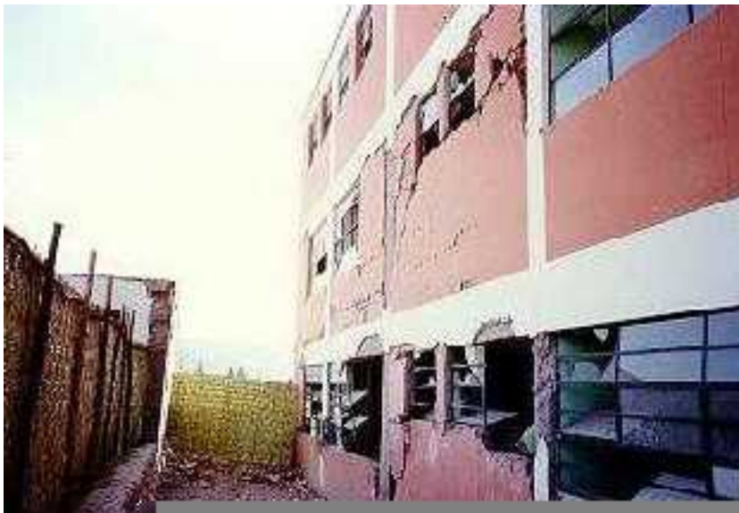
FIGURE 6: A Photograph Illustrating Typical Earthquake Damage
