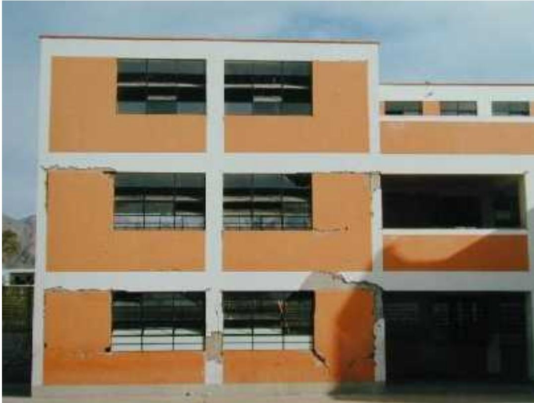
FIGURE 6: A Photograph Illustrating Typical Earthquake Damage (1996 Nazca earthquake)
