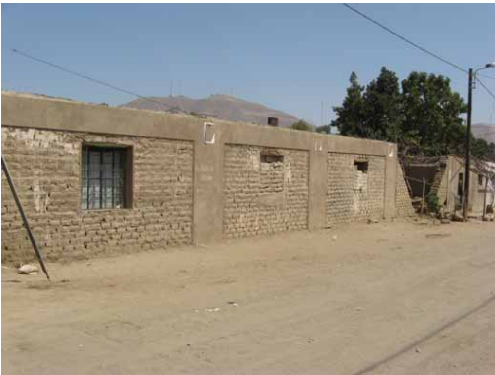
Fig. 3. This undamaged adobe house was reinforced with bands of wire mesh covered with sand-cement mortar. Vertical bands were placed at each wall intersection, and horizontal bands at roof level. Notice the collapsed unreinforced wall at the right.
