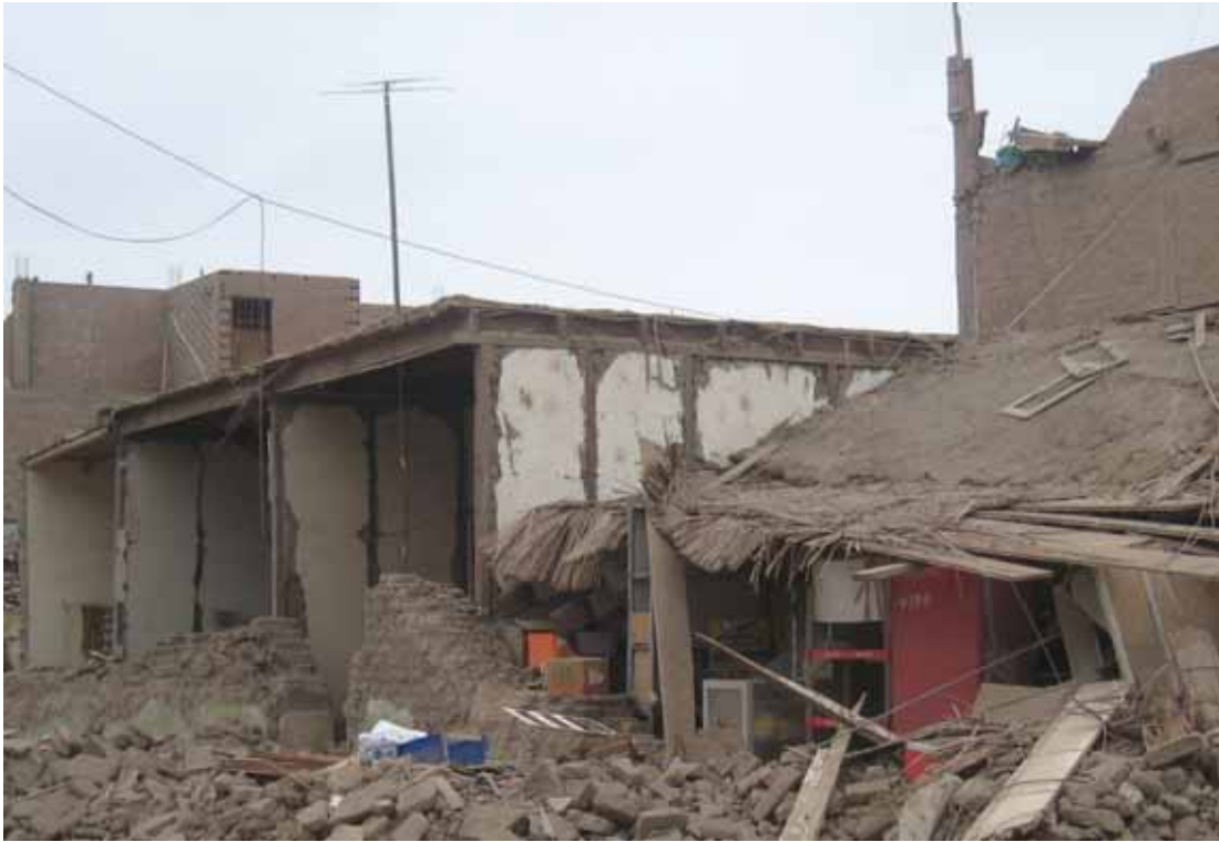
Fig. 2. Two collapsed adobe houses in Pisco. The roof joist of the house on the left are supported on the quincha partitions. The roof joists of the house on the right were supported on the façade wall, and thus collapsed with the façade. Notice the undamaged confined masonry house at left, and the collapsed masonry parapet on the house at the back right.
