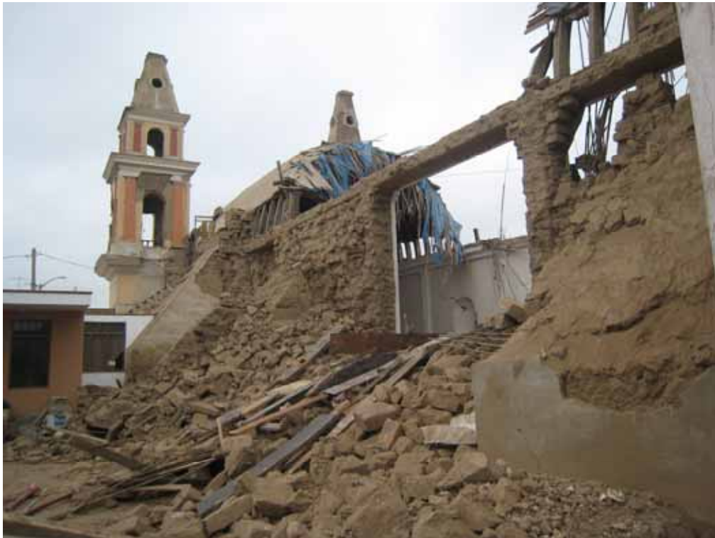
Fig. 4. San Luis Church. The lateral wall and its heavy abutments were practically torn down, presumably by the dynamic thrust of the collapsing vault. The towers are made of quincha and suffered little damage.
