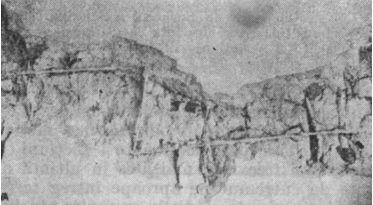
FIGURE 5D: Typical Earthquake Damage in RC Shear walls; note cracking in the construction joint (1977 Vrancea Earthquake)
