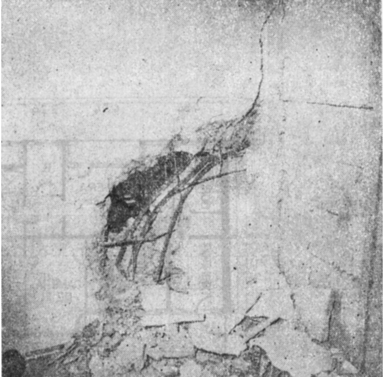
FIGURE 5C: Typical Earthquake Damage in RC Shear Walls (1977 Vrancea Earthquake)
