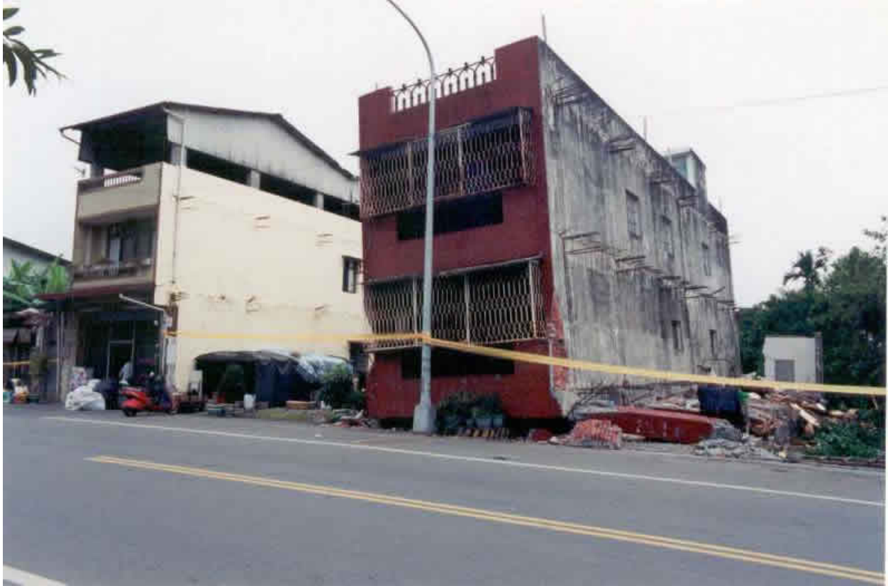
FIGURE 6B: Earthquake damage-Collapsed Three-story building in the 1999 Chi Chi earthquake (Source: EERI 2001)
