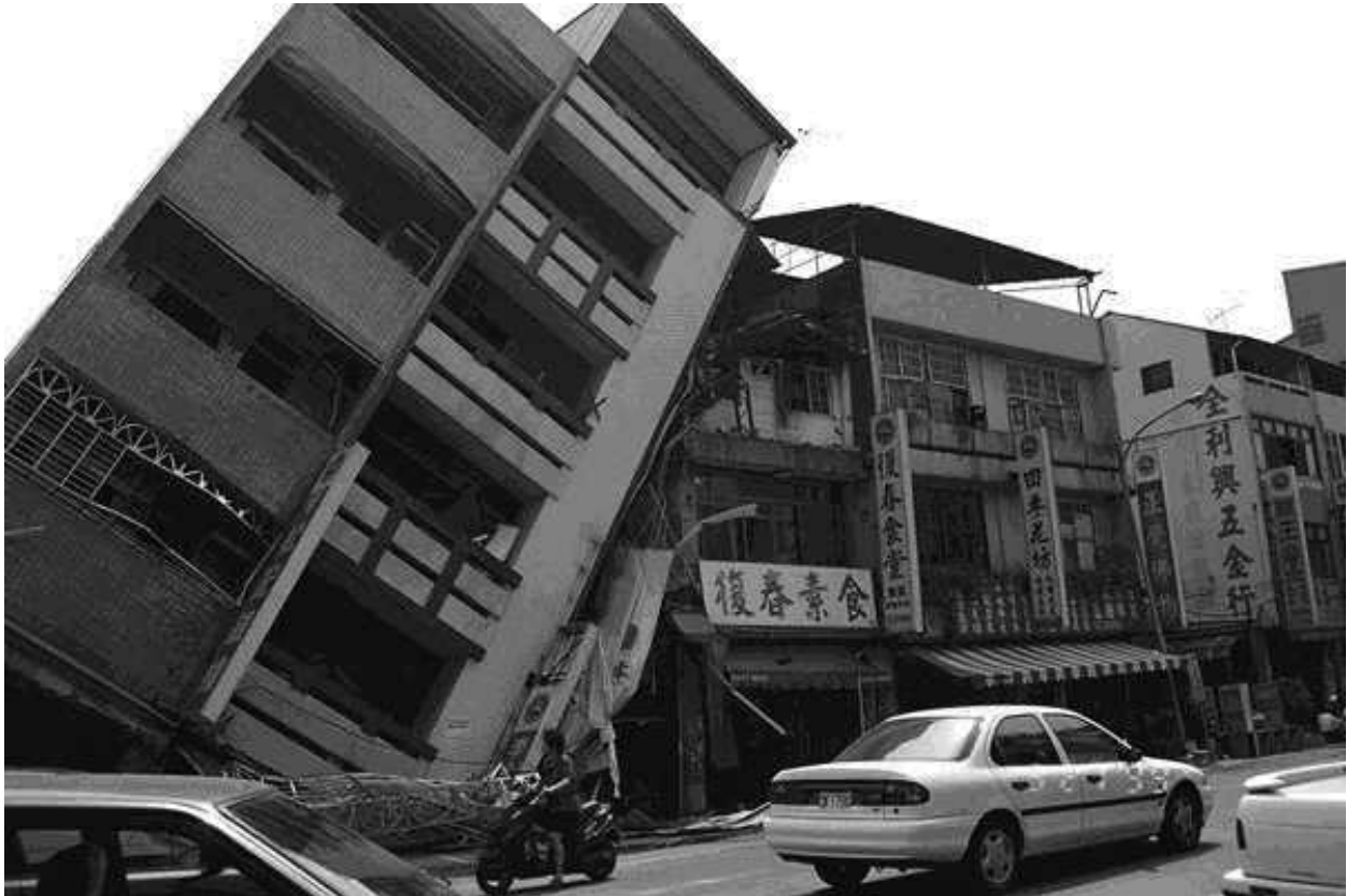
FIGURE 6F: Collapse of a Concrete Frame Building in the 1999 Chi Chi Earthquake (Source: EERI 2001)
