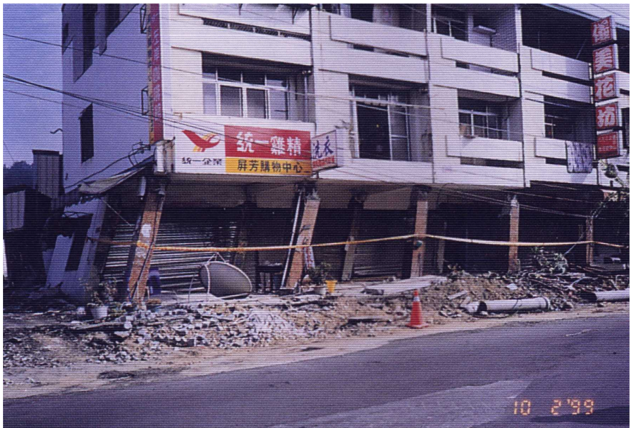
FIGURE 6A: A Photograph Illustrating Typical Earthquake Damage
