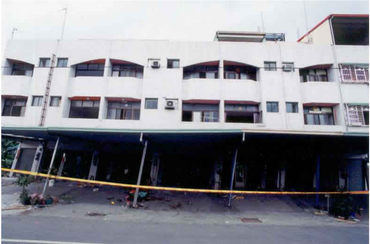
FIGURE 6C: Earthquake Damage - Partial Collapse of a Three-story building in the 1999 Chi Chi Earthquake (Source: EERI 2001)
