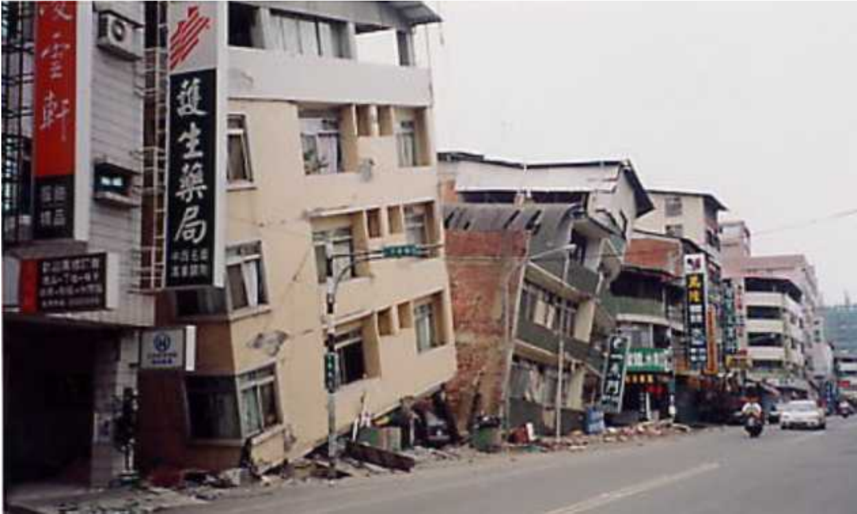
FIGURE 6A: A Photograph Illustrating Typical Earthquake Damage (1999 Chi Chi earthquake)
