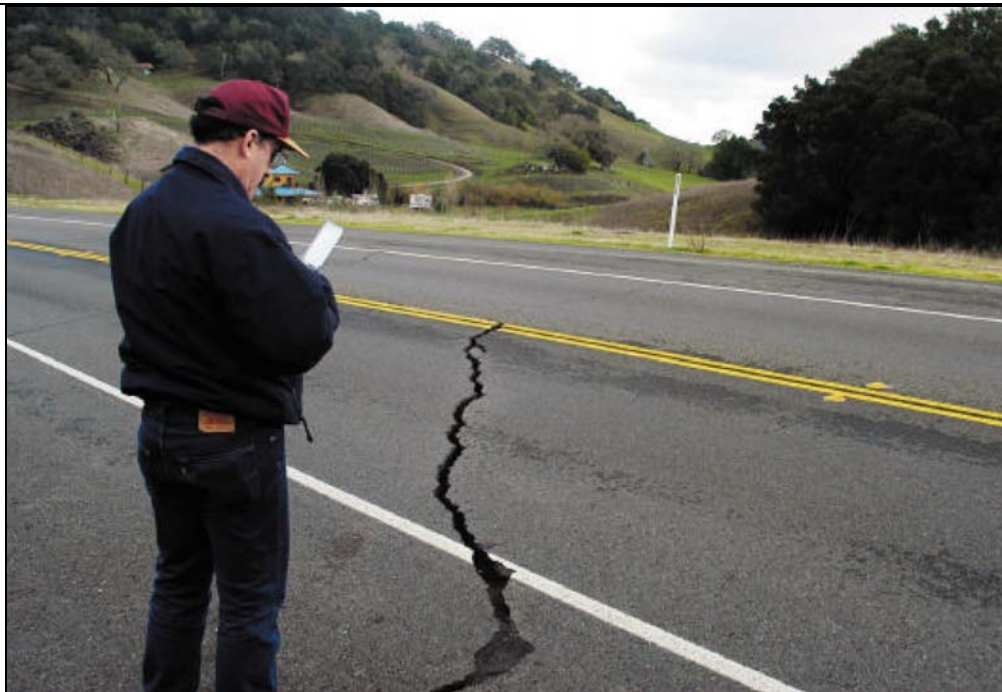
Lou Rosenberg (San Luis Obispo County Geologist) standing in front of damage to Highway 46.
