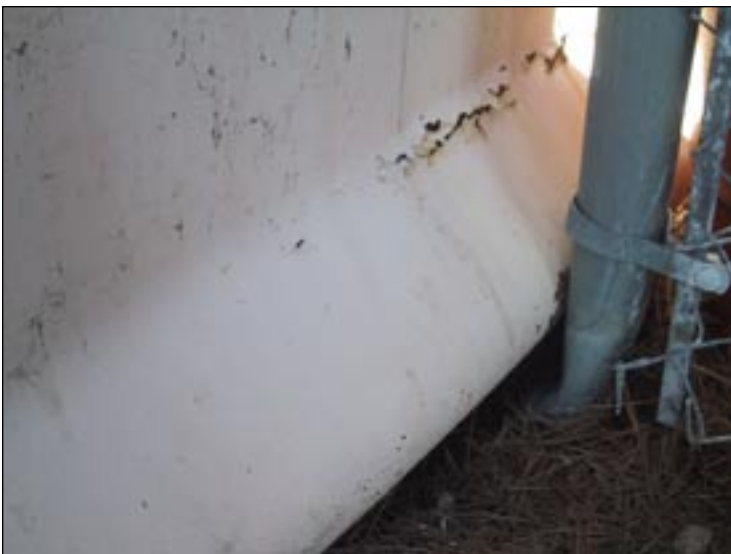
Figure 7. Buckle and fence post (photo Eidinger).
