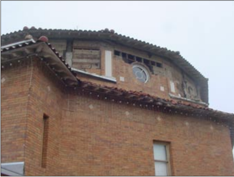
Figure 10. Atascadero City Hall facade damage (photo Lynn).
