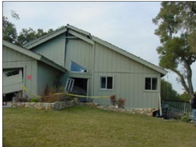
Figure 11. Residential collapse in Atascadero (photo Lynn).
