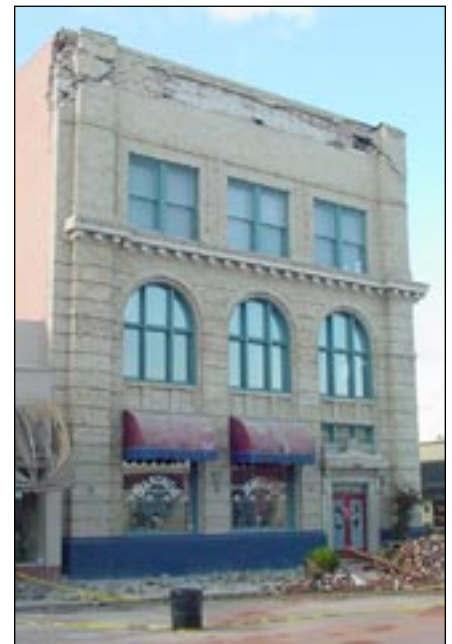
Figure 9. Nonstructural parapet and veneer brick damage (photo Lynn).
