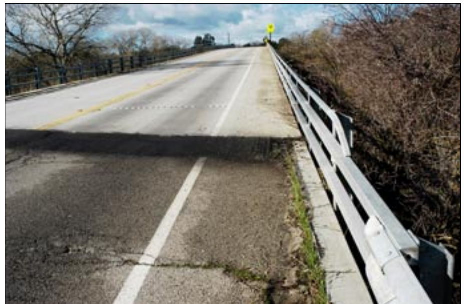
Figure 6. Templeton Road Bridge approach settlement (photo Yashinsky)
