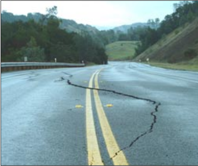
Figure 5. Seismic compression and slope instability along SR 46 (photo Chadwell).
