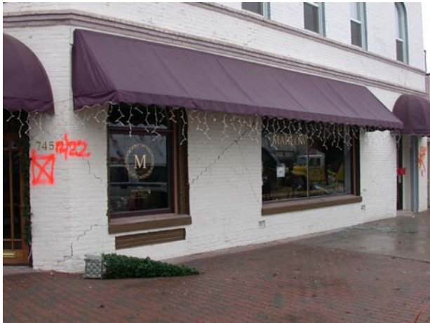
Figure 11. Crack pattern in the first story of the Marlow Interior building on the Park Street face (Picture by Sam Vigil).
