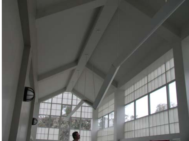
Figure 29. Damage to a light fixture in Recreational building on the Campus of California Polytechnic State University, San Luis Obispo (Picture by Rakesh Goel).
