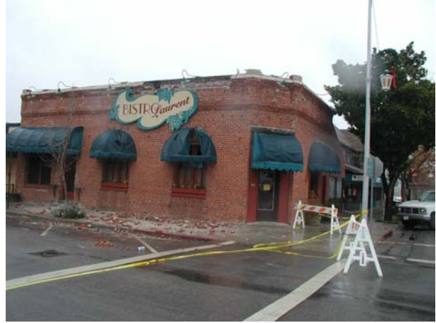
Figure 14. Minor peeling of bricks from the decorative parapet of the Bistro Laurent building on the corner of Pine and 12 th Streets in downtown Paso Robles (Picture by Rakesh Goel).
