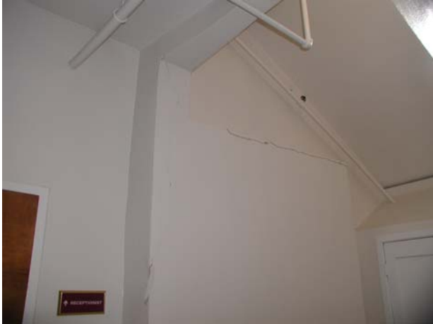
Figure 23. Typical cracks in the walls of Atascadero City Hall (Picture by Rakesh Goel).
