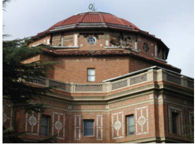
Figure 22. Peeling of brick façade from the rotunda of the Atascadero City Hall (Picture by Rakesh Goel).
