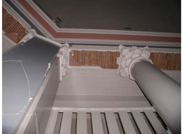
Figure 24. Peeling of plaster from ring beam of the rotunda of the Atascadero City Hall (Picture by Rakesh Goel).
