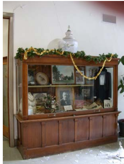
Figure 24. Damage in the lobby of the Atascadero City Hall (Picture by Sam Vigil).
