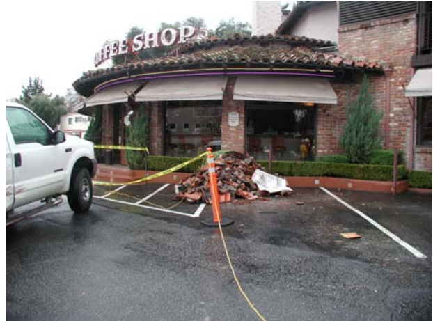
Figure 18. Loss of windows and roof tile in restaurant of the Paso Robles Inn (Picture by Rakesh Goel).
