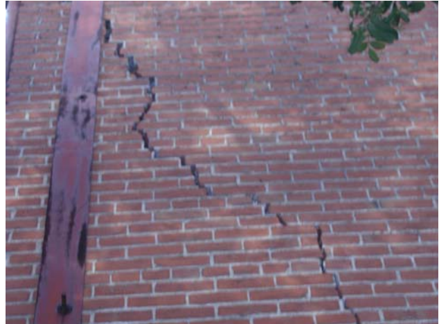
Figure 26. Cracks existing prior to the earthquake and attempt to retrofit on the south-west wall of the Ah Louis Store building (Picture by Rakesh Goel).
