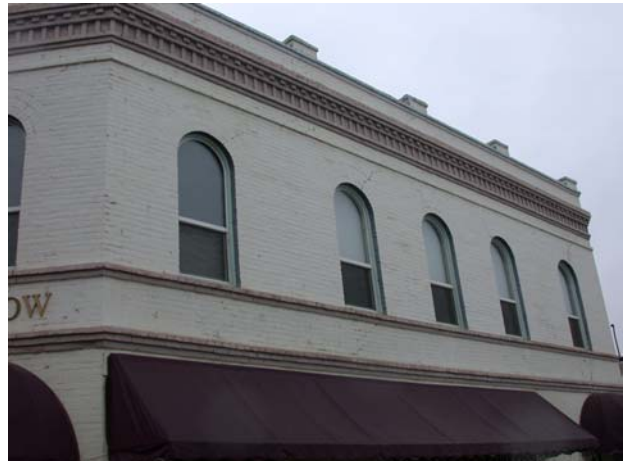
Figure 12. Crack pattern in the second story of the Marlow Interior building on the Park Street face (Picture by Sam Vigil).
