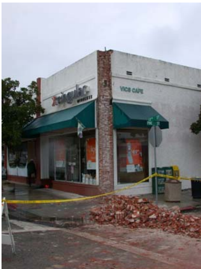
Figure 15. Damage to the Cingular Wireless building on the corner of Pine and 13 th Streets in downtown Paso Robles (Picture by Sam Vigil).
