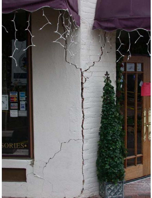
Figure 10. Large cracks at the corner of the Marlow Interior building (Picture by Sam Vigil).
