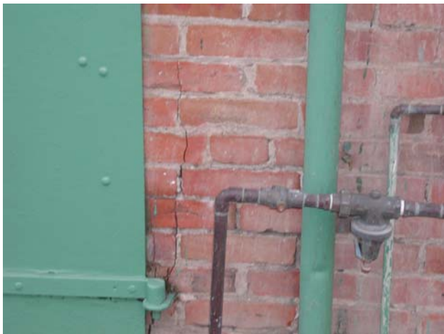
Figure 27. New cracks on north-east wall of the Ah Louis Store building (Picture by Rakesh Goel).
