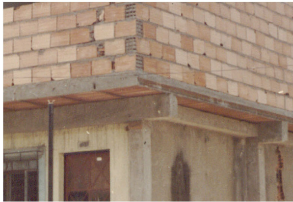
Inadequate connection between floor and frames
