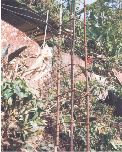
Ties and Stirrups widely spaced, 90 ° Anchorage hooks
