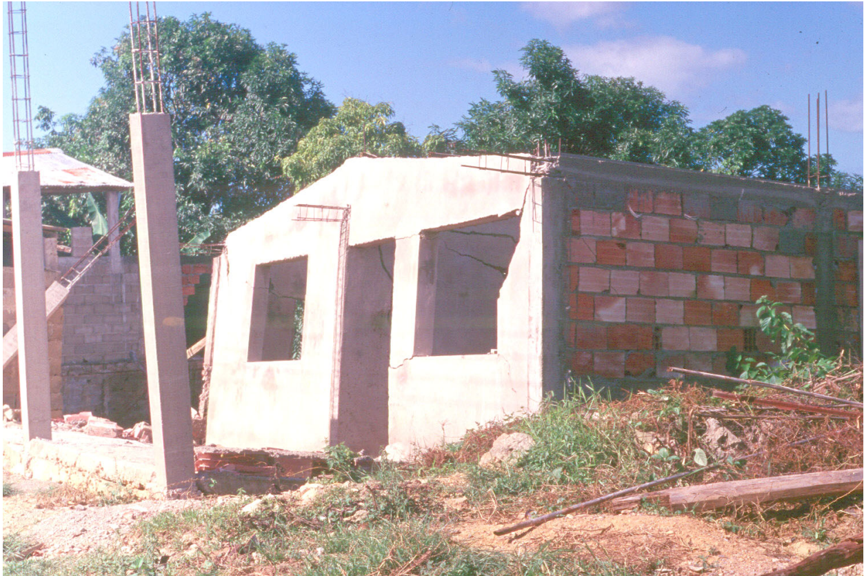
FIGURE 6: A Photograph Illustrating Typical Earthquake Damage (1997 Cariaco earthquake)
