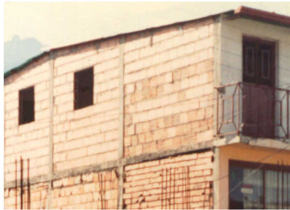
Inexistent Collar Beam
