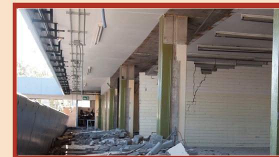
2010 El Mayor-Cucapah earthquake: Collapsed wall of the Engineering Building of the Universidad Autónoma de Baja California, Mexicali campus.
