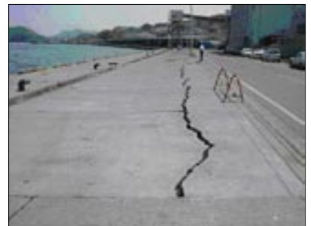
Damage caused by foundation settlement in Ofunato (photo courtesy of National Research Institute for Earth Science and Disaster Prevention).
