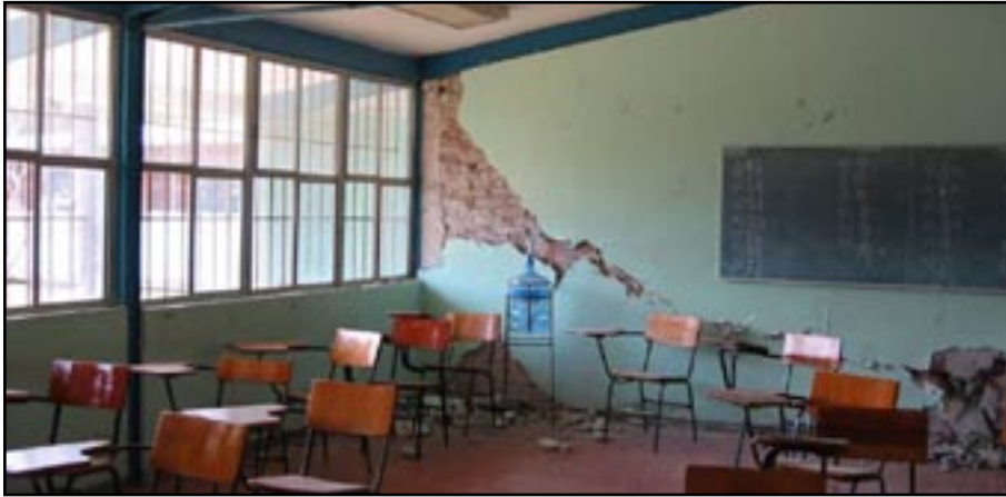
Figure 19 - Inclined cracking in an infill wall of a school building in the village of Ixtlahuacan. The structure of the school is made of light gage steel members.
