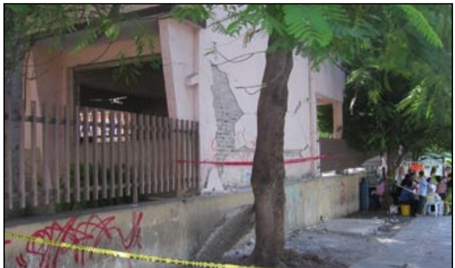
Figure 18 - Damage to a school building.
