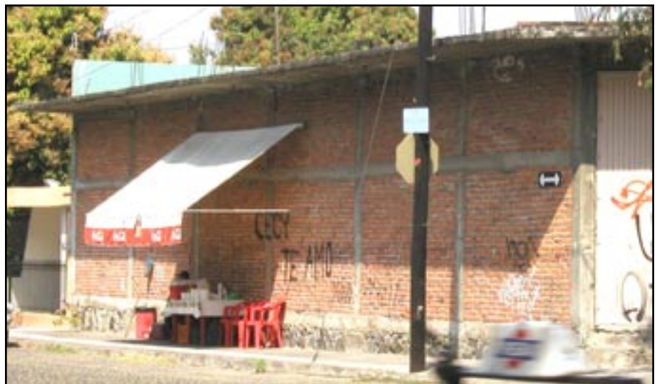
Figure 11 - A typical confined masonry structure, which performed well in the Tecomán earthquake.
