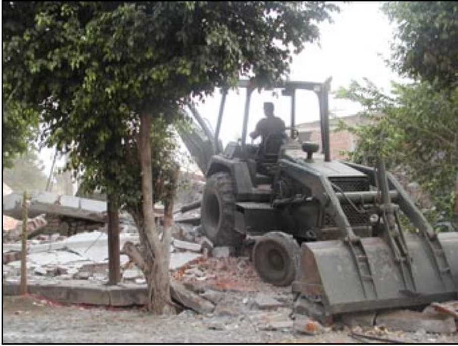
Figure 17 - Demolition by the Mexican military of adobe structures categorized as totally damaged.
