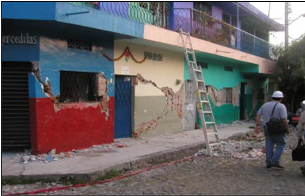
Figure 12 - Typical damage to unreinforced masonry structures.
