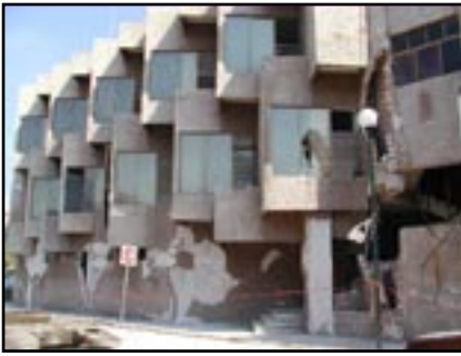
Figure 13 - Example of lack of structural continuity of vertical and horizontal elements.
