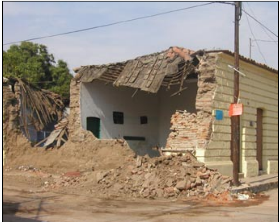
Figure 14 - Typical damage to adobe structure at the corner of a block.
