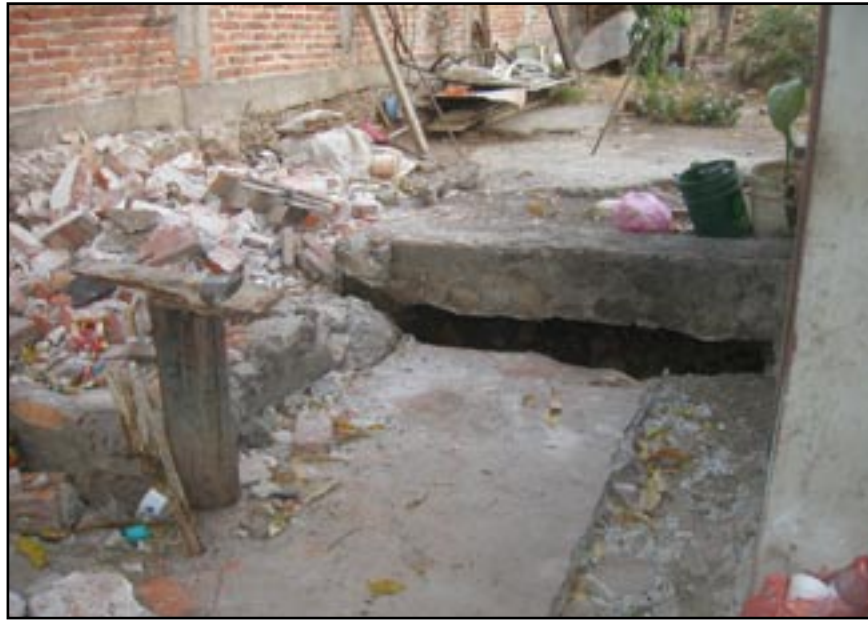
Figure 5 - Large settlements in a house in the San Isidro neighborhood, possibly due to collapse of poorly consolidated fills.
