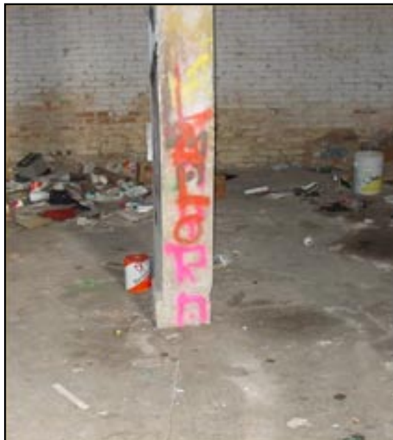
Figure 7 - Bearing-capacity failure in Colima. The column dropped through the floor of the structure, ultimately settling about 0.3 m.
