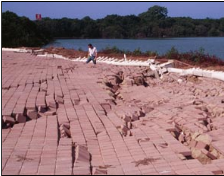
Figure 6 - Liquefaction-induced lateral spread in Manzanillo (for scale, each paving block is 0.20 m square).
