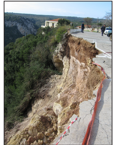
Landslide at Mitata (Photo: E. Lekkas).
