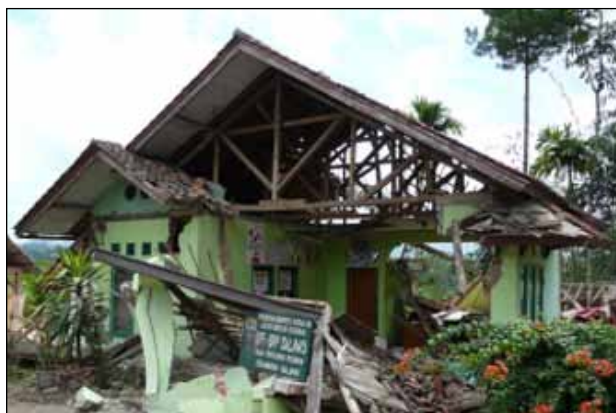
Figure 2. A building with confined masonry walls failed due to low-quality materials and poor workmanship.
