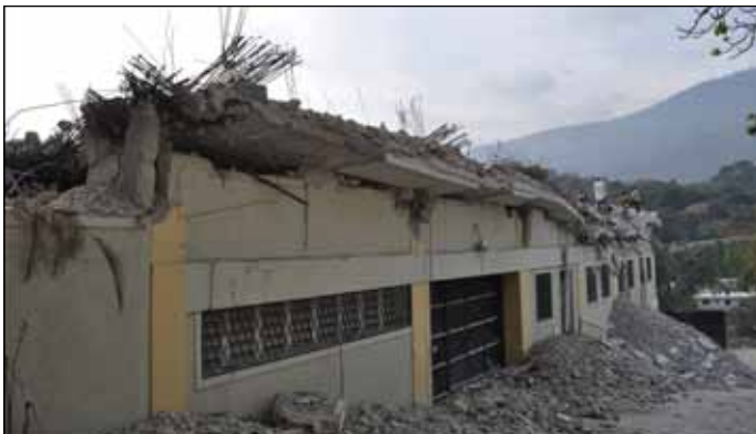
Damage and partial collapse at UN Development Programme Annex (photo: Ayhan Irfanoglu).
