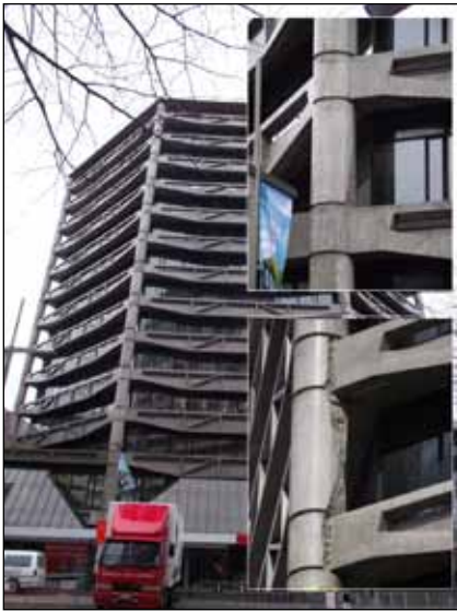
Figure 11. Perimeter column spalling throughout the height of a reinforced concrete frame with perimeter precast trusses in West-Pac building in downtown Christchurch (photo: Dusicka)
