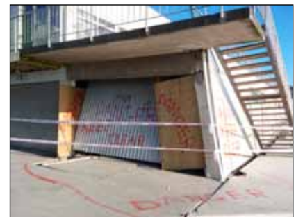
Figure 10. Damage to a reinforced concrete building from lateral spreading at a site near the Avon River (photo: Roeder)
