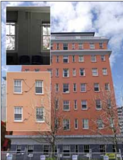
Figure 8. Shear cracks in perimeter masonry walls of an eight-story reinforced concrete frame building in downtown Christchurch (photo: Dusicka)
