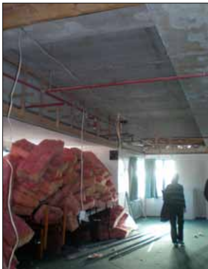
Figure 17. Nonstructural damage at the University of Canterbury: fallen ceiling tiles and hangers (photo: Comerio)
