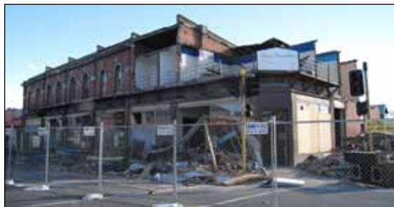
Figure 20. The building housing Angus Donaldson, and other businesses on Colombo St. in Sydenham, is cordoned off two weeks after the quake (photo: Arendt).
