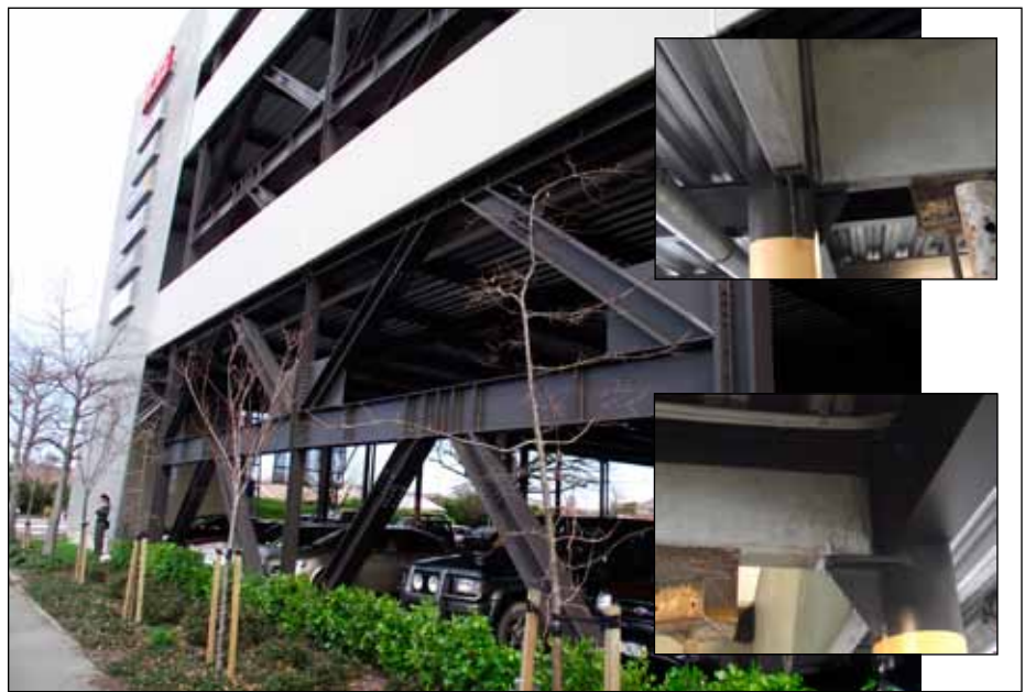
Figure 9. Cracks at beam seats of gravity load precast members used in parking garage, along with undamaged eccentrically braced frame lateral system in Christchurch area (photos: Dusicka).
