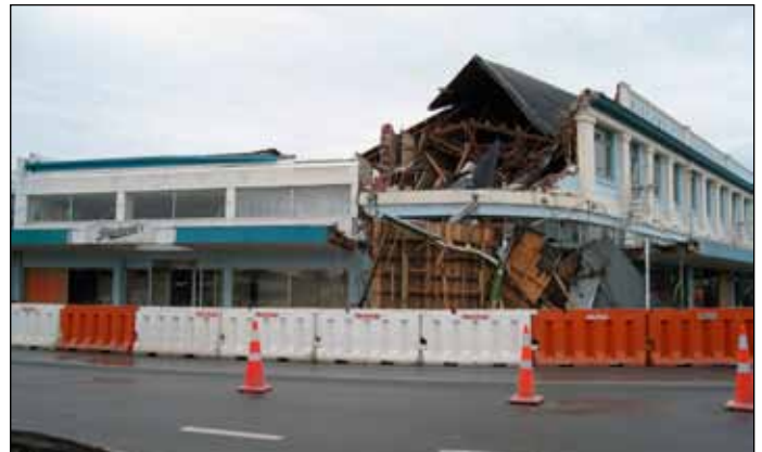
Figure 16. Blackwell's Department Store on William Street in Kaiapoi suffered extensive structural damage (photo: Arendt)
