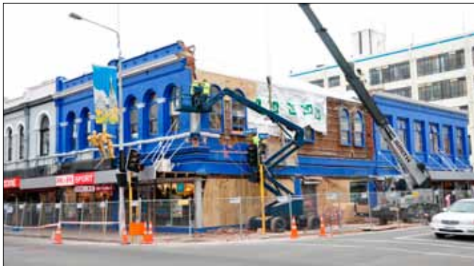
Figure 15. This corner building had braced parapets only fronting on the main street, left. The secondary street wall separated from the roof, falling onto the street and sidewalk below (photo: Turner).
