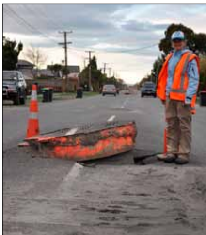
Figure 4. Uplifted manholes along Lower Styx road. (photo: Green)
