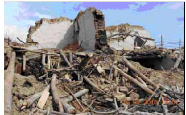
Destroyed two-story adobe house.
