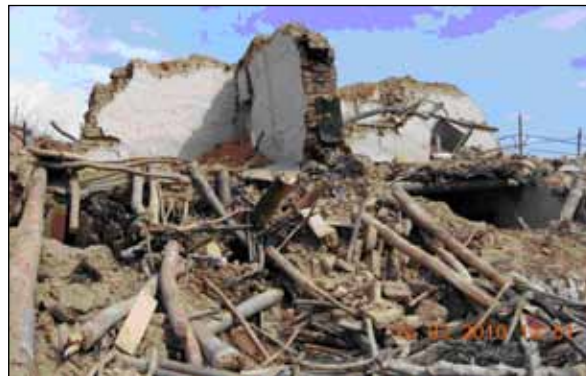
Destroyed two-story adobe house.
