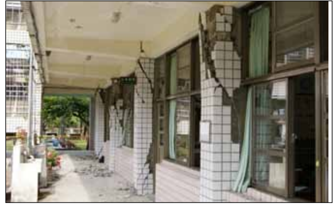
Typical damage to corridor columns.
