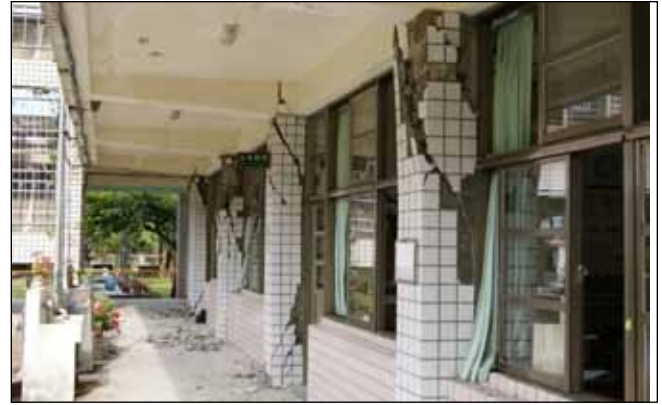
Typical damage to corridor columns.
