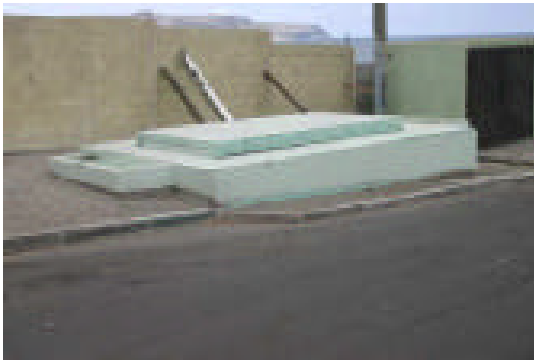
Treatment plant and surge chamber of outfall sewer.
