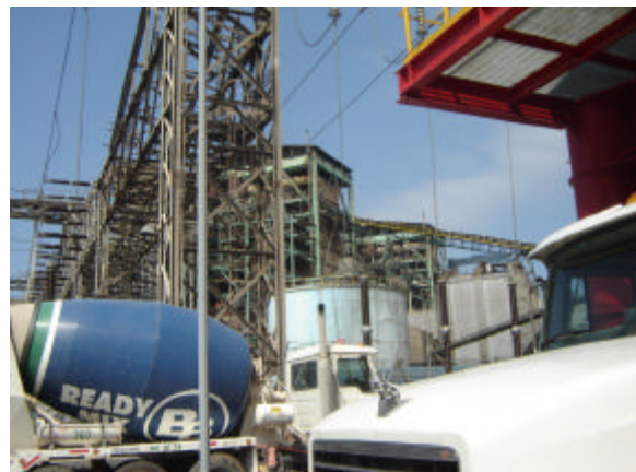
View of undamaged thermoelectrical plant near the station located on rock in Tocopilla.
