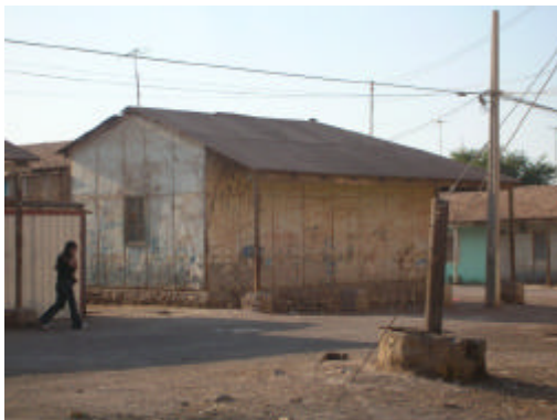
c) Wooden frame with low quality concrete infill in Maria Elena.
