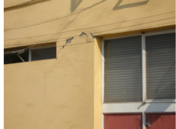
Moderate damage in short columns of the Gobernacion building.
