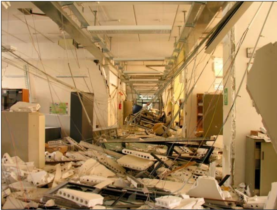
Figure 15. The interior of the City Planning Offices in L'Aquila. Note that the building exterior has very minor detectable damage.
