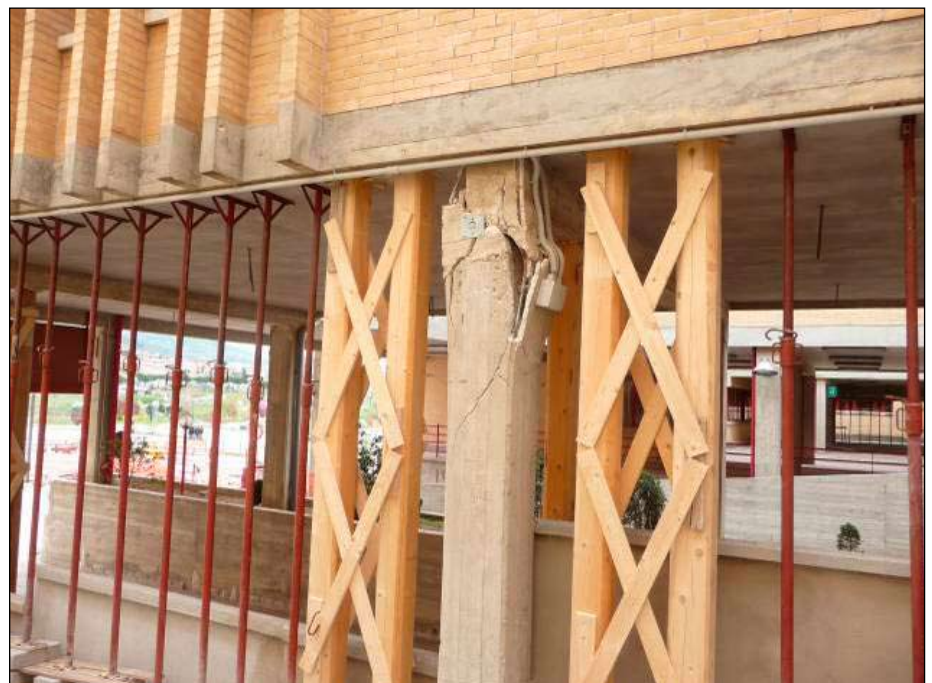
Figure 16. Column damage at hospital entry structure; no tie reinforcement is evident.
