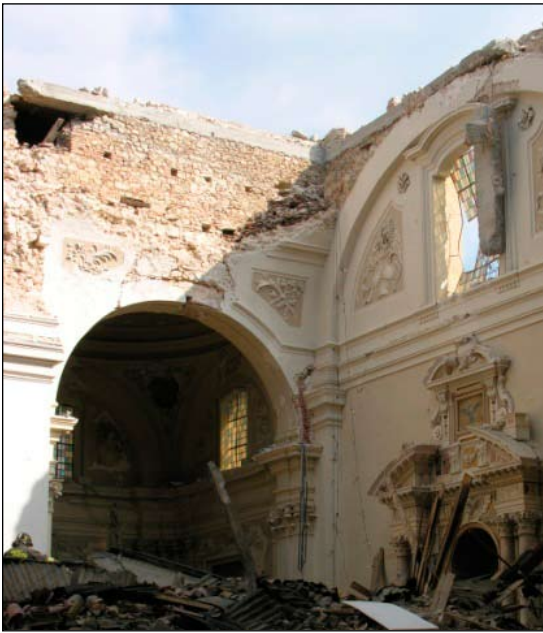
Figure 10. Roof and cupola collapse in the Santa Maria di Collemaggio Abbey in L'Aquila. The reinforced concrete ring beam did not prevent the collapse of the cupola.
