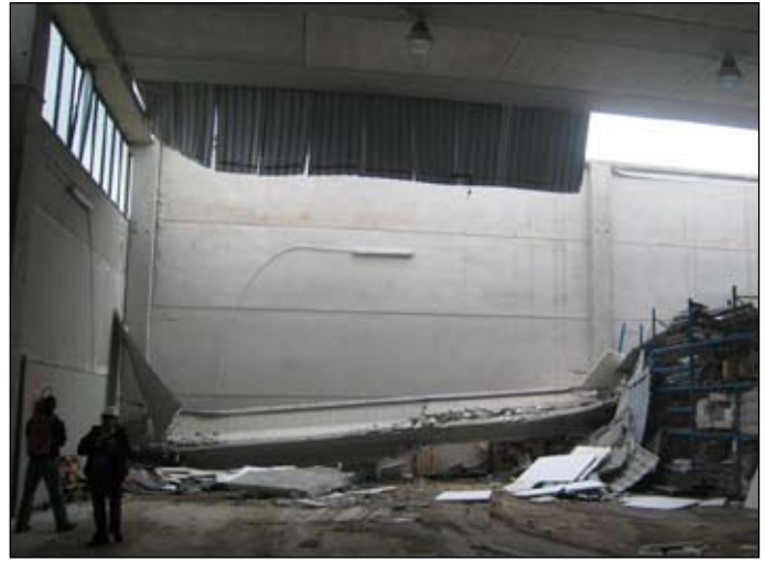
Figure 18. Partial collapse of the roof.
