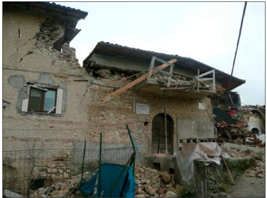
Figure 8. Collapse of a masonry building in Temperra with concrete ring beam retrofit.
