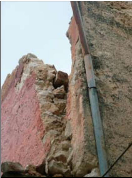
Figure 7. Detail of 18th century wall-strengthening system, where no ties connect the beam to the wall.
