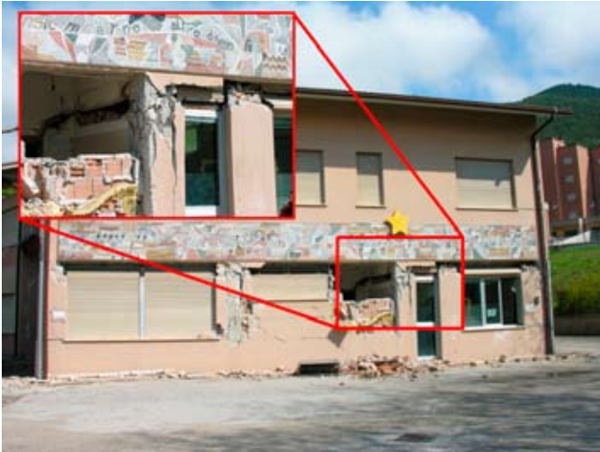
Figure 17. Extensive damage to the elementary school in Pettino.
