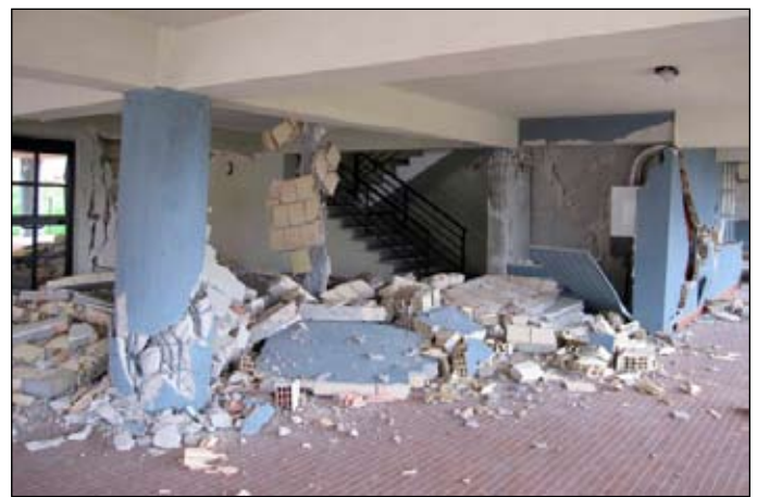
Figure 14. Core shear wall with extensive structural damage and failure in a modern RC building in Pettino.
