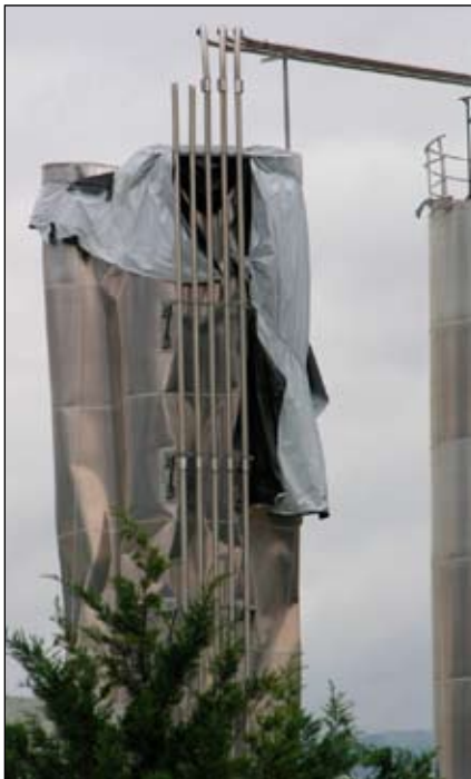
Figure 19. Extensive damage at one silo.
