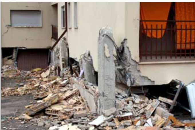
Figure 13. Soft-story collapse in Pettino. Two of four almost identical structures collapsed.
