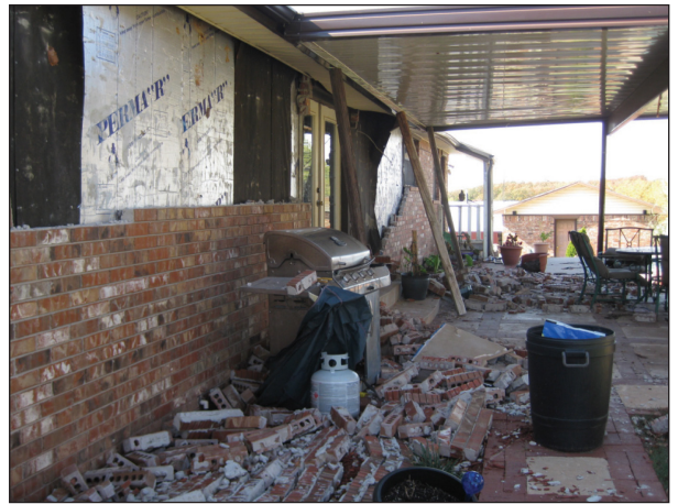
Figure 1. A severely damaged home in Meeker, Oklahoma.
