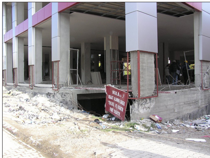
Figure 1. A heavily damaged six-story building in Ercis. The structural layout resulted in excessive floor torsion. The flexible joist floors with block infills had cracks around columns at every floor level. The columns failed at the base of the ground story (photo: A. Irfanoglu).
