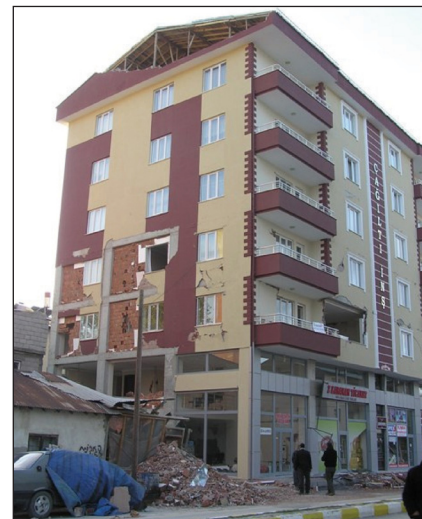
Figure 2. A newer building in Ercis with a typical tall ground story and mezzanine level for commercial use (photo: A. Irfanoglu).
