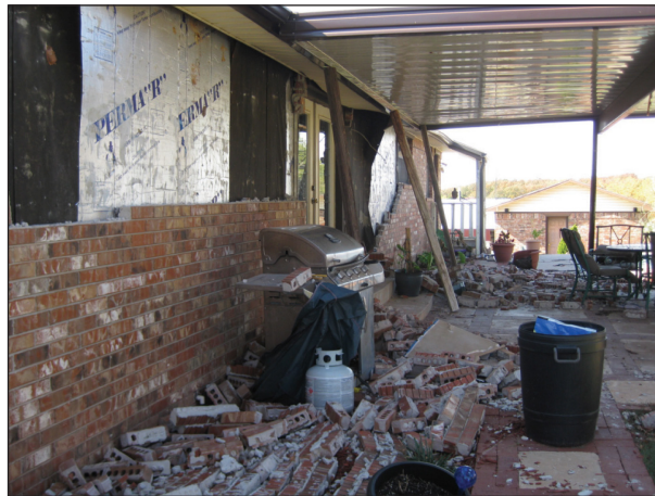
Figure 1. A severely damaged home in Meeker, Oklahoma.
