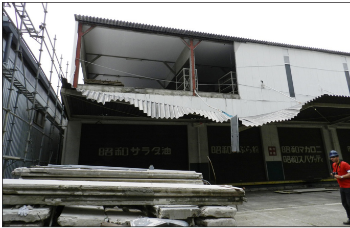
Figure 22. ALC panels fallen from a two-story office-and-warehouse building.
