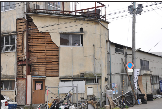
Figure 20. Cladding damage to older residential building.
