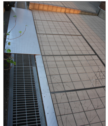
Figure 41. Damage to moat cover of base isolated building.
