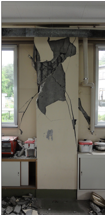
Figure 4. Junior high school built in 1966, located 10 km N. of Kuriyama. Wing walls along the exterior, nominally reinforced and cast eccentrically with columns, induced shear failures that penetrated through the columns.
