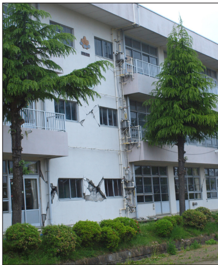
Figure 3. Elementary school in Sukagaya. Column damage at classrooms depended on presence or absence of cast-in-place infill at the base. Infill creating captive column with integrated wing walls caused shear failures.
