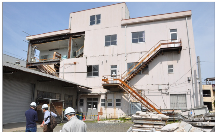
Figure 21. ALC panels fallen from a three-story office building.
