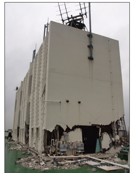
Figure 13. Severe damage to two-story reinforced concrete mechanical penthouse.
