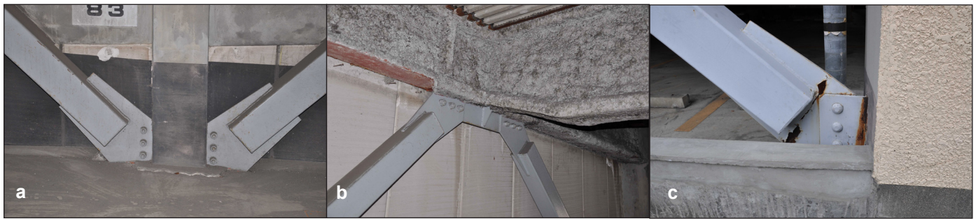
Figure 17. Typical gusset plate design details and failure modes in garage 16a: (a) foundation uplift, (b) welded stiffener, (c) gusset plate yielding.
