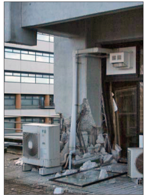
Figure 9. Damage to columns at tower-podium transition (photo: M. Motosaka).
