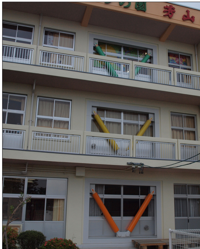
Figure 7. Elementary school approximately 1 km east of Koriyama. Stiff retrofits, such as diagonal steel bracing and infill shear walls, were effective at preventing structural damage.
