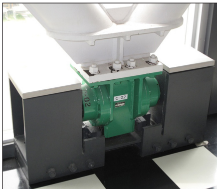
Figure 42. Tohoku Institute of Technology Building B10 supplemental damping.
