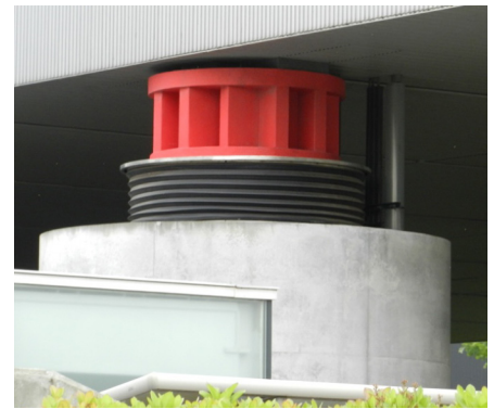
Figure 39. ▶ One of six lead rubber isolators supporting the main building.
