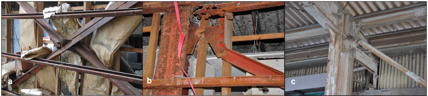
Figure 19. Typical failure modes in old Japanese construction design: (a) lateral torsional buckling, (b) net section fracture, (c) net section fracture, (d) panel zone yielding.
