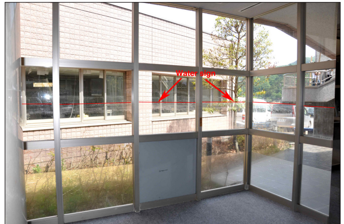
Figure 26. Water signs, first story of Onagawa hospital.
