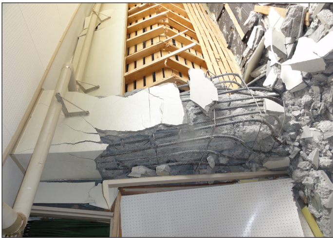
Figure 5. Junior high school located 10 km north of Koriyama. Interior column below end of discontinued shear wall above.
