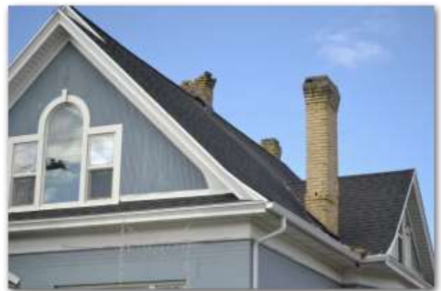
Partially Collapsed Chimneys
