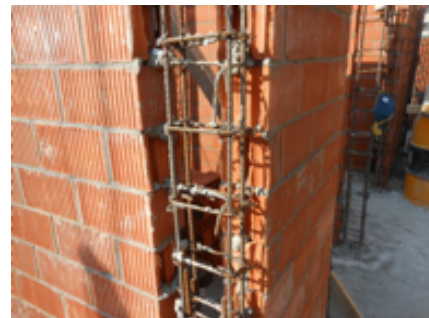
Figure 2. Wall intersection showing horizontal steel dowels with 90 degree hooks as an alternative to tothing
