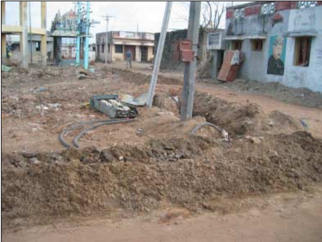
Figure 2. Damaged telephone cross connect box for the village. (Tang)
