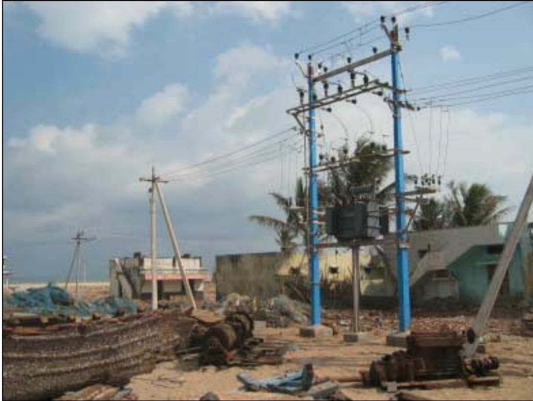
Figure 3. New transformer and new poles for power distribution (Tang)
