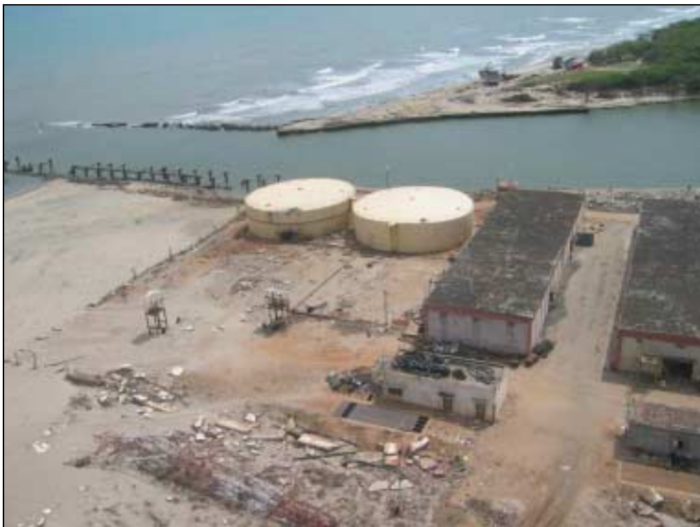
Figure 8. Damaged pier – for loading cooking oil to the tanks (Tang)
