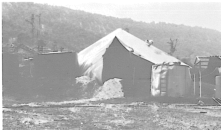
Fig. 6 Destroyed oil storage tank at Salado Pump Station. Landslide debris ruptured tank, spilling 4,500 barrels of crude oil over pump station.
