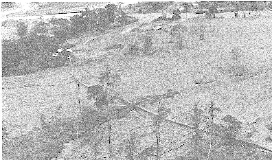
Fig. 5 Trans-Ecuadorian Pipeline deformed by broad debris flow into Coca River.
