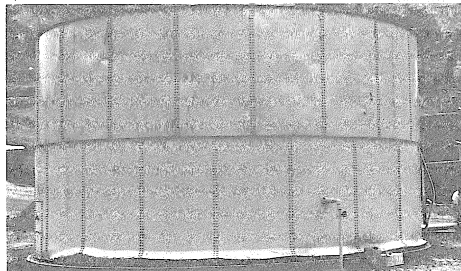
Fig. 7 Damaged water storage tank at Salado Pump Station.
