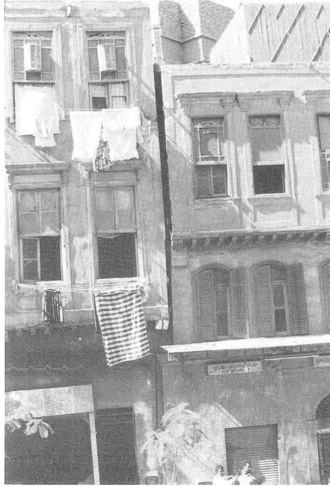
Building separation at expansion joints and tilting of some buildings.
