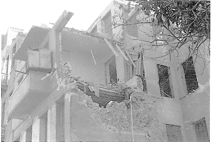
Old Cairo - Heavy damage to stone bearing wall buildings with unanchored wood roofs
