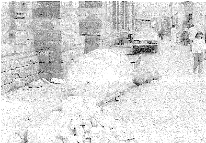
Ornate top of minaret that failed during the earthquake (Al Hanafi Mosque).
