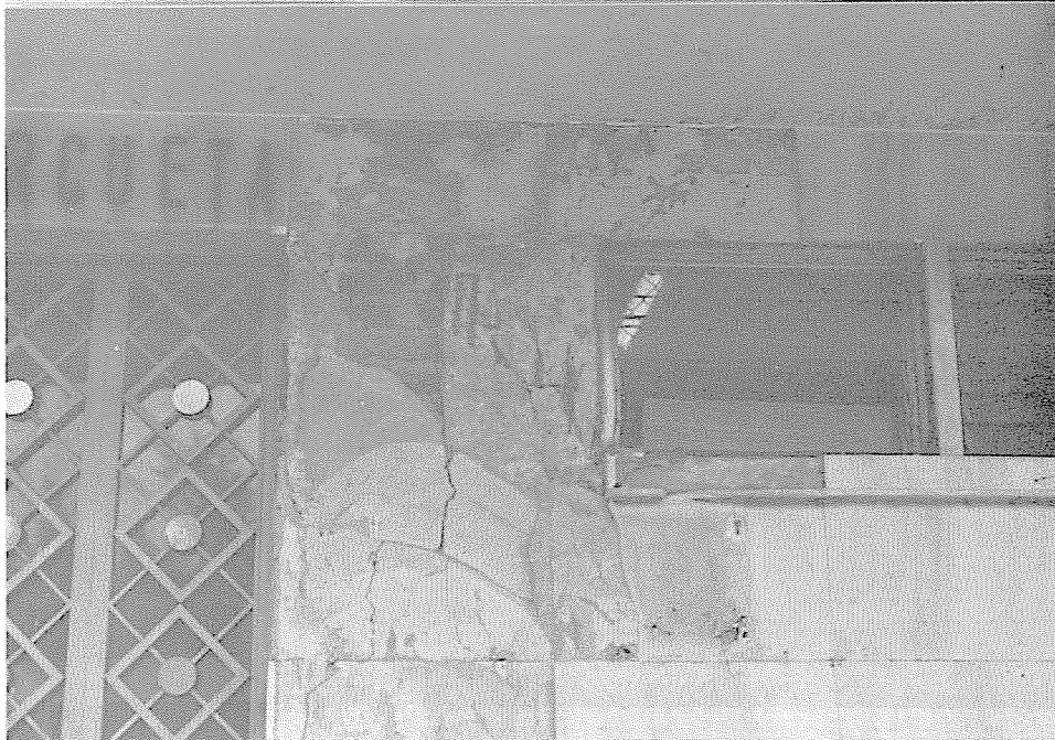
Building No. 13 Detail of Column Damage
