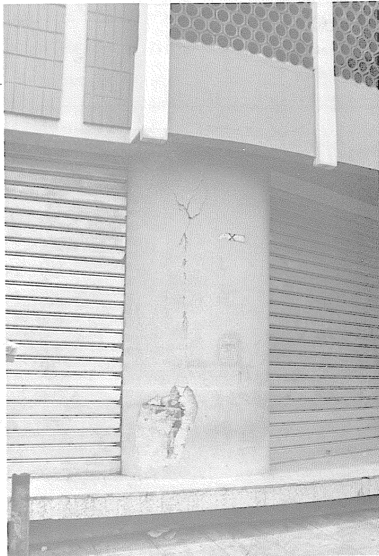
Building No. 16 Detail of Column cracking in 1st Story column
