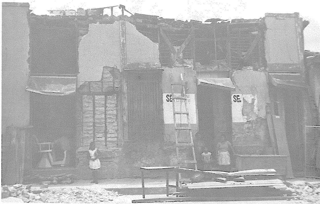
Severely Damaged 2-Story House in Ahuachapan -- Wattle Construction
